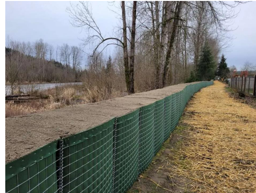
Completed A Street HESCO barrier on the right bank of the White River in Auburn, looking downstream. Credit: King County
