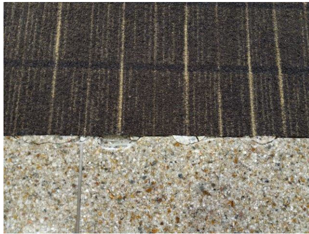
Detail of terrazzo damage
