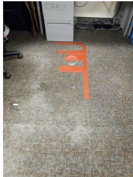
Detail of TSA office carpet damage
