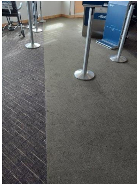
Gate 3 carpet damage
