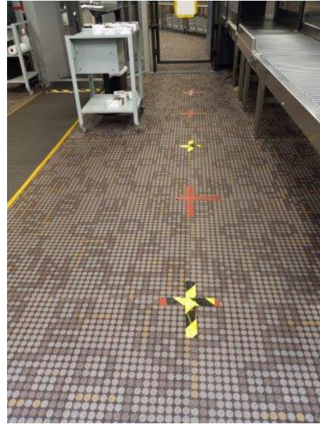
TSA screening carpet damage
