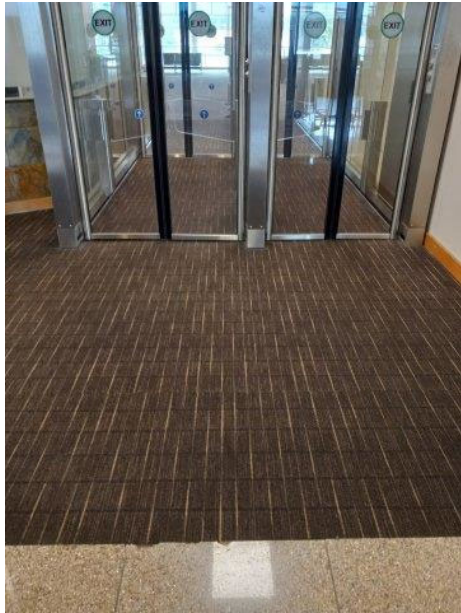
Terrazzo damage at exit lanes
