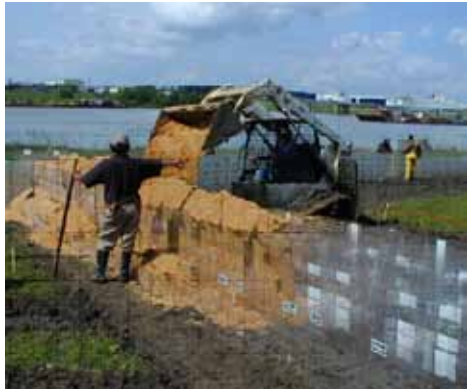
Rapid Deployment Floodwall
