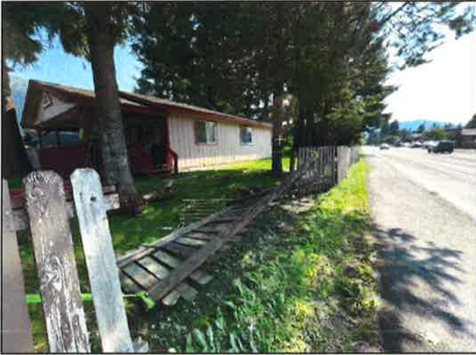
Image #5: Flood damage from flowing water down Riverside Drive.
