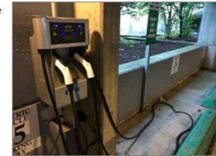
Marine Parking Garage EV Charging Station
