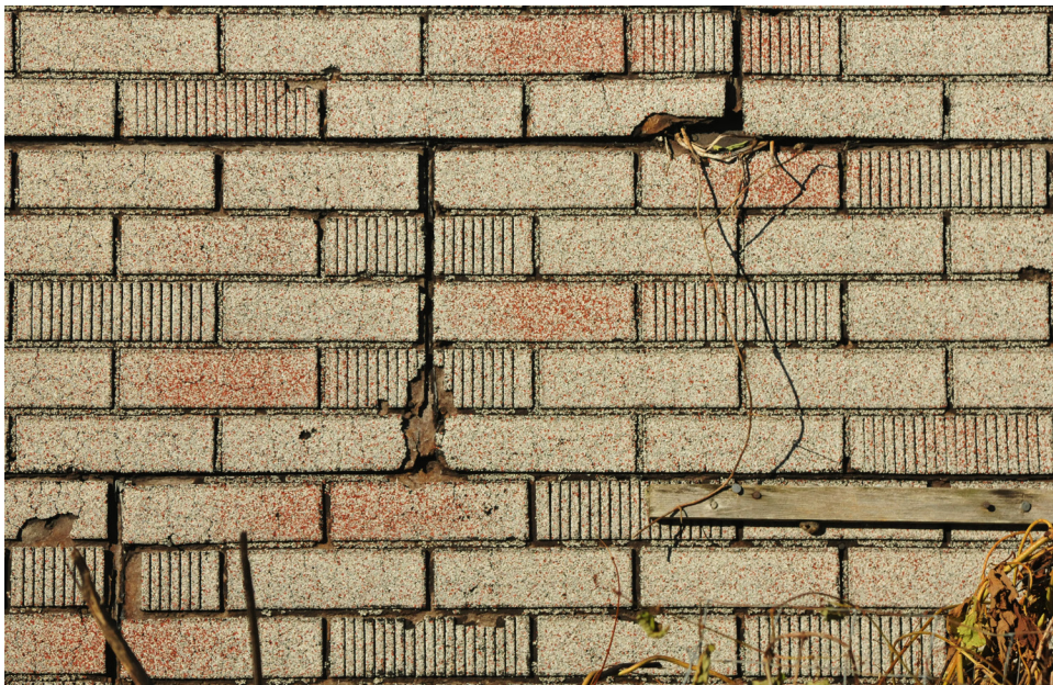
Asphalt-shingle siding covers the original clapboard siding. Therefore the residence does not retain the key exterior materials dating from the period of its historic significance. Edward Webster House, 2023
