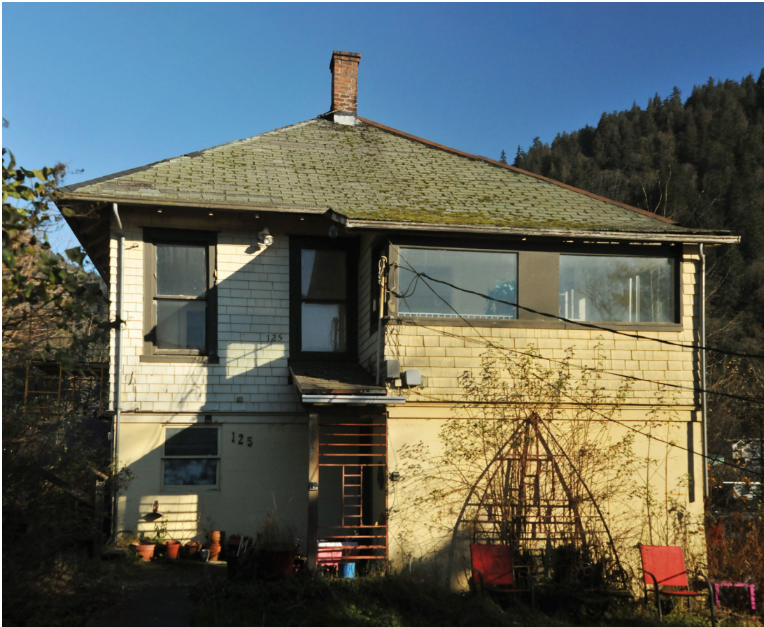
West Facade. Cedar shingles cover original clapboard siding. The large, picture windows in the upper left are part of the open porch that was enclosed in the 1950s. Worthen-Hurley House, 2023
