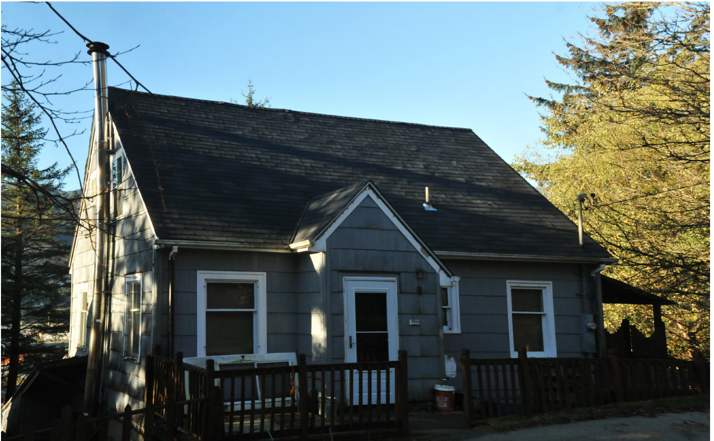
East Facade. Contemporary windows replace originals. Contemporary wooden deck added. Martin-Johnston House, 2023
