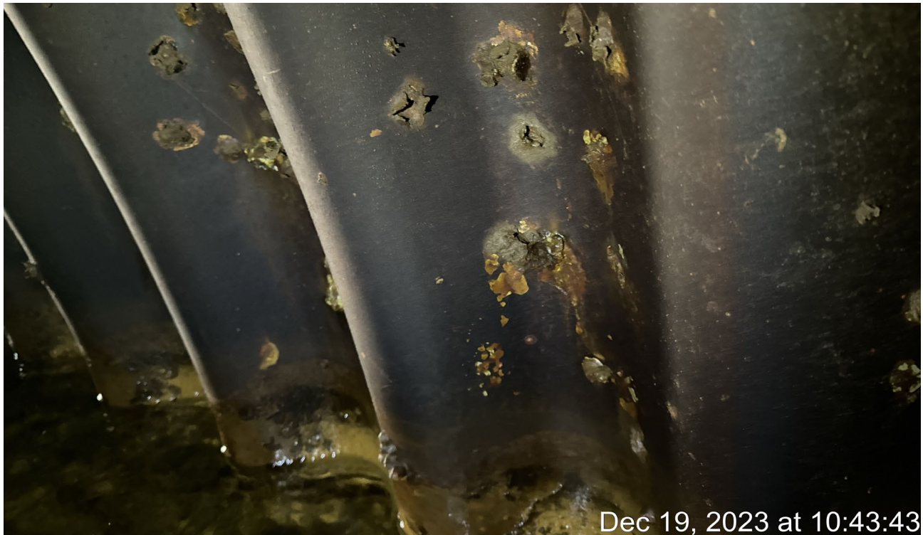
Photo 01: Heavy pitting and holes as observed on a portion of the half-arch culvert sidewalls.
