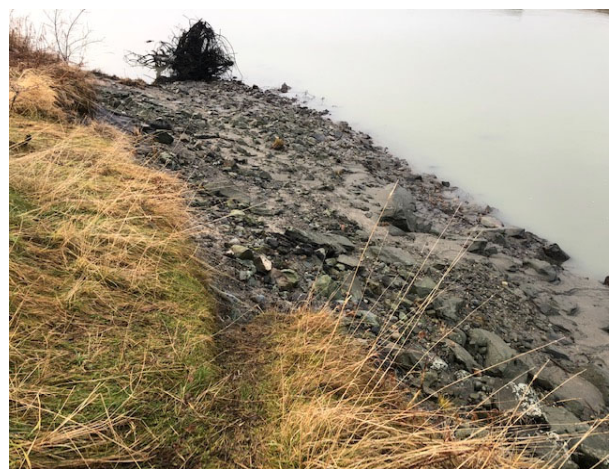
Photo 02: Damaged area looking down river. Rock loss ends near the tree root ball shown at top of photo.
