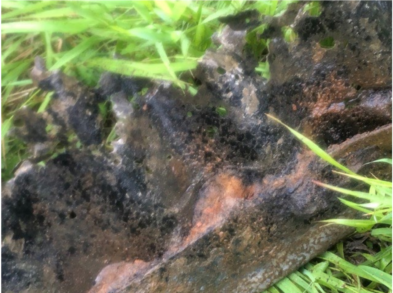
Heavy pitting along the lower – submerged – edge of the old culvert.
