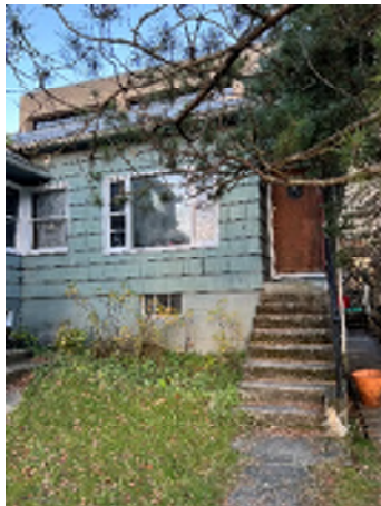
Figure 7-3. Moss on the Concrete Stairs.
