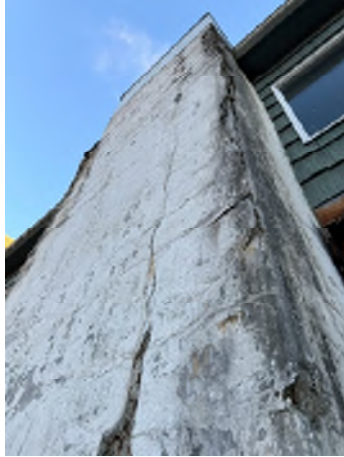
Figure 7-13. A Long Crack Up the Side of the Chimney.
