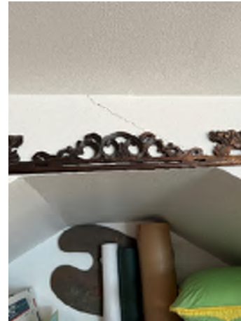
Figure 7-36. Sheetrock Cracks Through the Unit.
