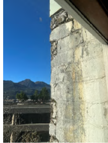
Figure 7-14. Concrete Falling Off the Side of the Chimney.
