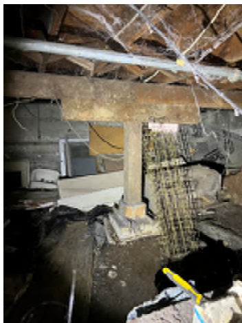
Figure 4-35. Column Sitting Directly on the Foundation With No Positive Connection to the Concrete or to the Beam.
