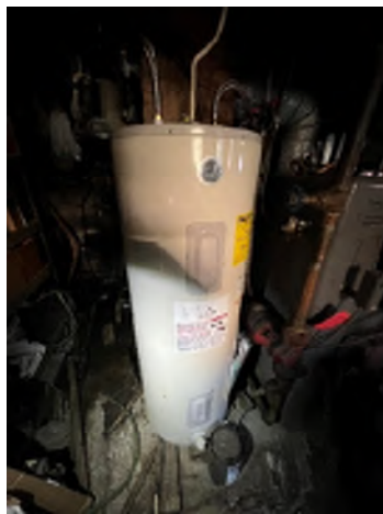
Figure 6-26. No Seismic Strapping on the Water Heater.
