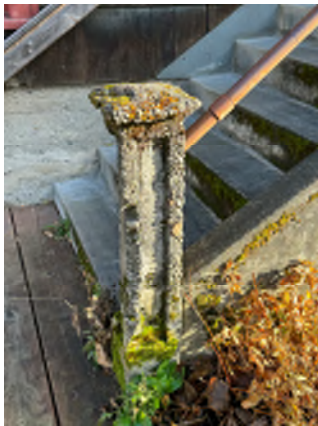
Figure 6-3. Damaged Concrete Post.
