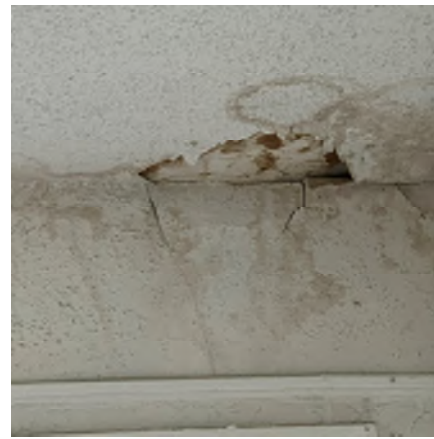
Figure 2-18. Ceiling Paint Is Cracked and Falling From the Water Infiltration. How extensive the water damage is or if there is mold is unknown without a destructive investigation.
