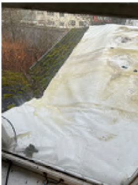
Figure 4-11. Tarp Covering the East Roof. There are known leak issues at the interface of the lower roof and wall.
