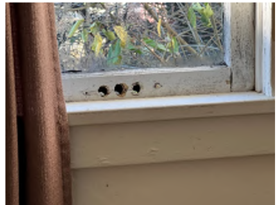
Figure 3-34. Mold and Holes in the Windowsill. The holes can lead to water infiltration.
