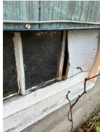
Figure 7-16. A Basement Broken Window, Which Is Not Adequately Sealed, That Can Allow Water or Animals Inside.
