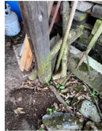
Figure 7-28. Moss Growing on Main Column Supports That Are not Pressure Treated. These columns can rot quicker untreated.
