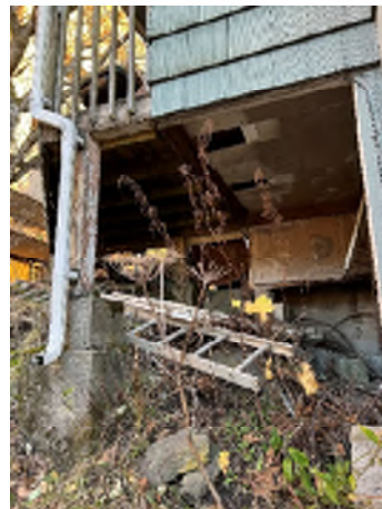
Figure 7-18. Missing Soffit Panels. The column is sitting on a concrete pile.
