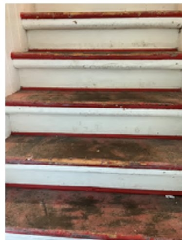
Figure 4-18. Steps Leading to the Second Floor Are in Poor Shape.
