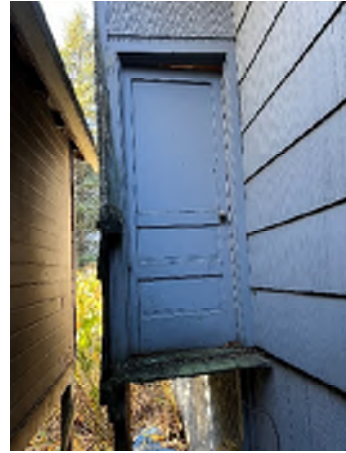
Figure 3-14. A Door Without Stairs Approximately 6 Feet Above the Ground. Some of the framing around the door is rotten.
