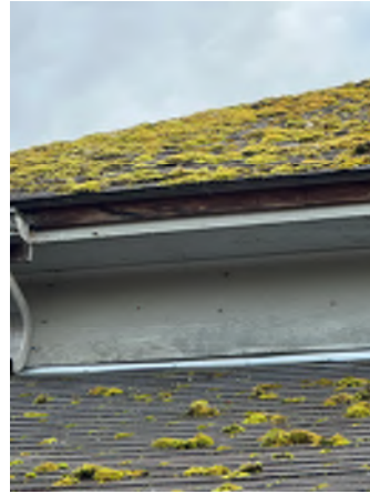
Figure 4-2. Exposed, Rotting Wood on the Eave.
