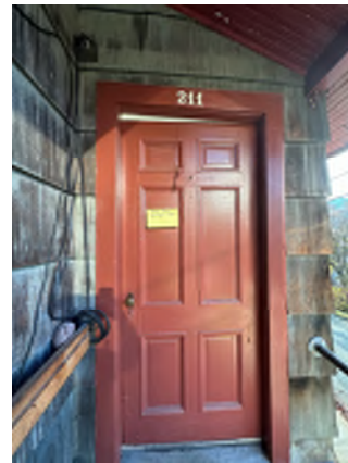
Figure 6-4. Large Gap Between the Door and Doorframe.
