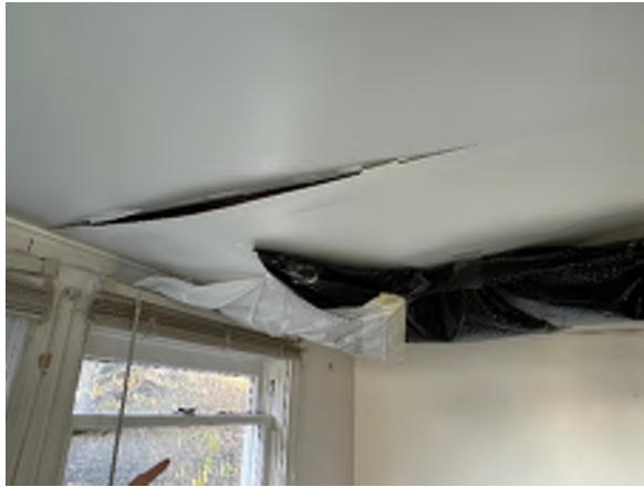
Figure 3-31. Ceiling Damage From a Roof Leak.
