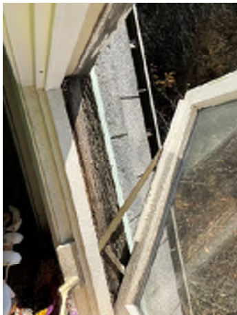
Figure 7-35. Rot Under Some Windows.
