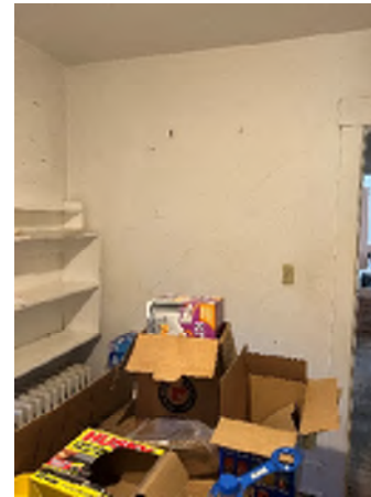
Figure 3-22. Wall Cracks Extending Diagonally Across the Entire Wall.
