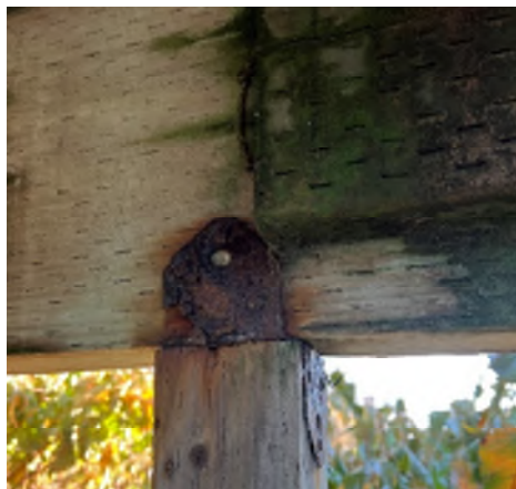
Figure 1-3. Rusty Hardware Connections on the Deck Framing.
