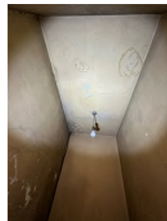
Figure 4-30. Cracking on the Ceilings and Walls and Signs of Water Damage.
