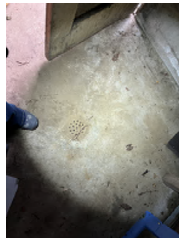
Figure 4-36. Drain Leads Directly Under the Foundation, Potentially Undermining the Foundation.
