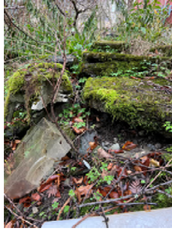
Figure 5-8. Undermined Walkway on the West Side of the Building.
