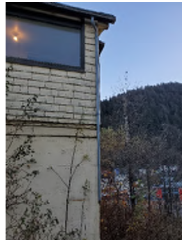
Figure 2-4. Drainage Pipe Ends Abruptly Mid-Air and Not Directing Water Away From the Foundation.
