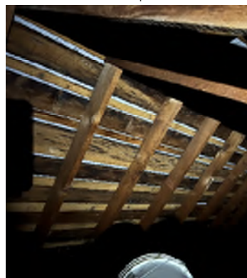
Figure 2-16. Indications of Previous Leak Repairs. Water infiltration can cause the structural members to rot. The roof rafters and site built trusses are under sized for current snow loads.
