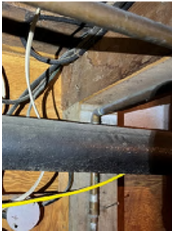
Figure 2-37. Columns Are Toe-Nailed at the Top to the Beam. No positive connection at the base of the column to the concrete exists.
