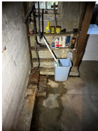
Figure 7-47. Multiple Signs of Water on the Basement Floor. There is a small trench for water around the perimeter.
