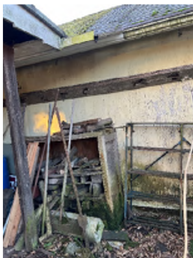
Figure 5-17. Gutter Drainage Splashed on the Garage and Caused Significant Moss to Grow and the Plywood to Rot.
