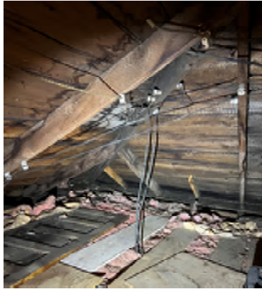
Figure 4-13. Cut Rafter Member and Extensive Water Damage From Past Events.
