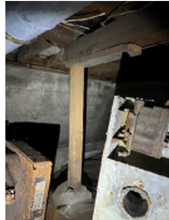
Figure 7-49. A Large Shim at the Top of the Column.
