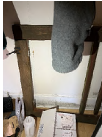
Figure 3-36. Sheetrock Crack in the Closet and Mold on the Baseboard.
