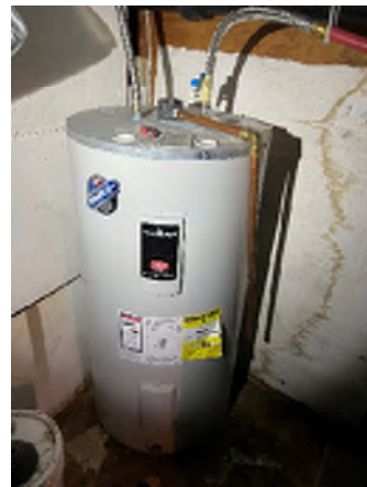
Figure 2-36. No Seismic Strapping Around the Water Heater.
