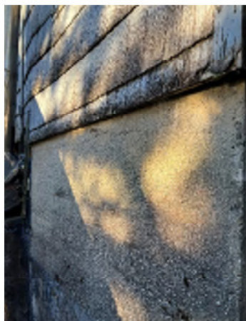
Figure 3-17. Long Crack at the Top of the Wall.
