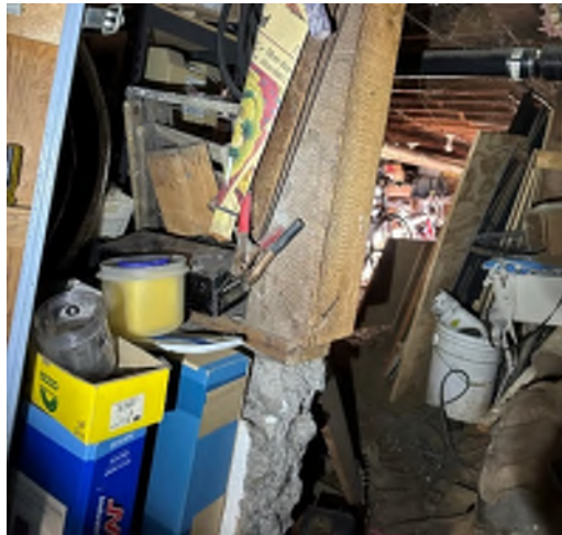
Figure 6-24. Wood Post Supported Eccentrically by Stem Wall With a Chunk of Concrete Missing Directly Below the Post.
