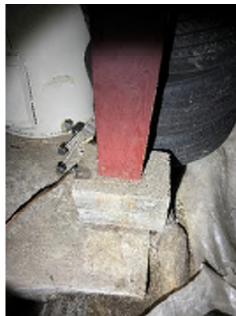
Figure 7-50. The Column Is on a Concrete Block That Is Not Sitting Fully on the Concrete Below.
