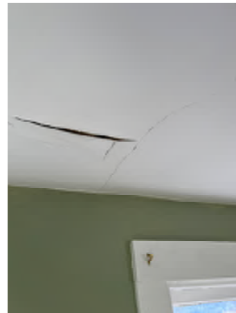
Figure 4-16. Cracked Sheetrock and Peeling Paint on the Ceiling.
