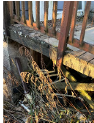
Figure 3-2. Drainpipe Is Disconnected and the Deck Framing Appears Rotten.
