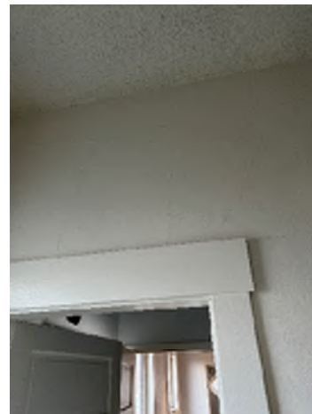
Figure 2-20. Sheetrock Cracks on the Wall in the Bathroom.
