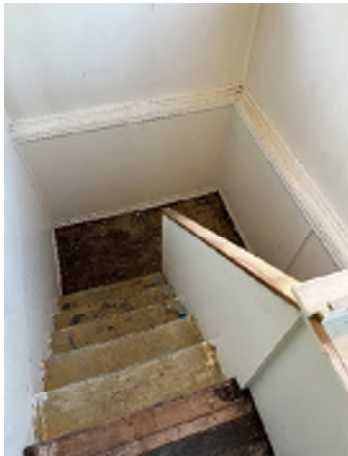
Figure 2-25. Much of the Flooring Was Removed, Leaving the Subfloor Unprotected.
