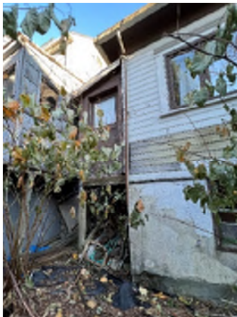
Figure 1-9. A Door More Than 6 Feet Above Ground With No Stairs.
