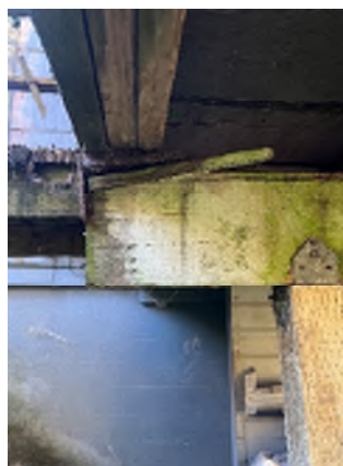
Figure 3-6. The Beam Supporting the Deck Is Shimmed Likely Due to Rot. No connection exists between the beam to deck framing.
