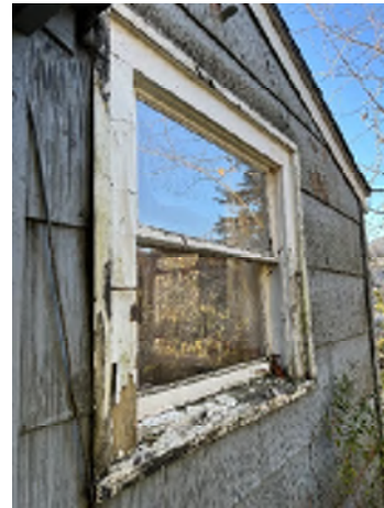
Figure 3-10. Rotten Windowsill and Siding in Poor Condition.
