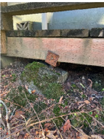
Figure 7-23. A Rotated Walkway Support Connector.
