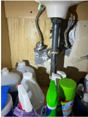
Figure 7-31. An Upper-Level Sink Leaked.
