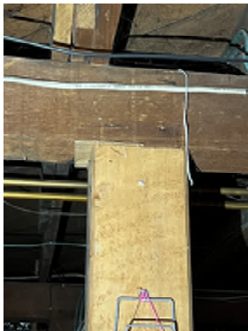
Figure 5-29. Shimmed Column With No Positive Connection to the Beam.
