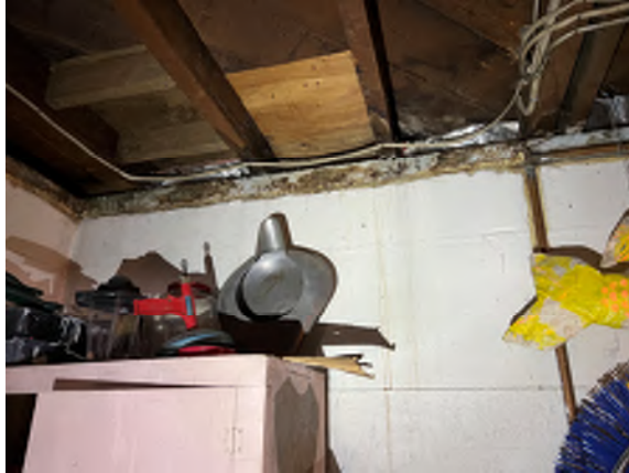
Figure 5-31. Water-Damaged Insulation and Water Marks Running Down the Concrete Basement Wall.
