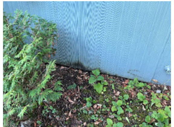
Figure 7-4. Soft Wood at the Base of the Siding.
