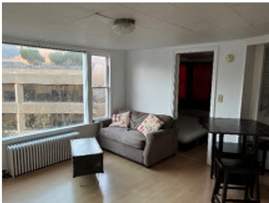
Figure 7-41. Finishes Appeared to Be in Good Condition.
