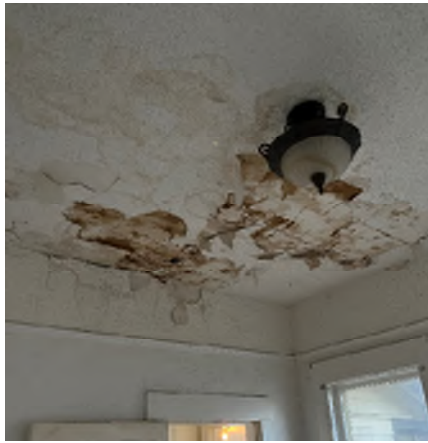
Figure 2-17. Significant Water Damage to the Ceiling Below the Roof Leak. The light fixture was not tested because of signs of water infiltration.
