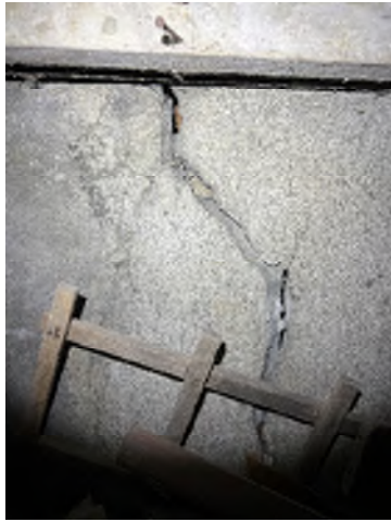
Figure 1-13. Visible Wood Framing in the Deep Crack Where Water Infiltrates the Basement.
