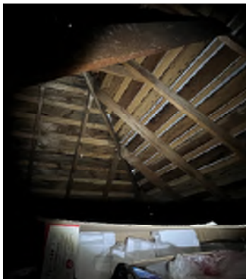
Figure 2-15. Daylight Is Visible Through Holes in the Northwest Corner of the Roof, Which Allows Water to Penetrate the Roof. This is the cause of the water damage seen on the ceiling of the second level. A roof replacement is in progress.
