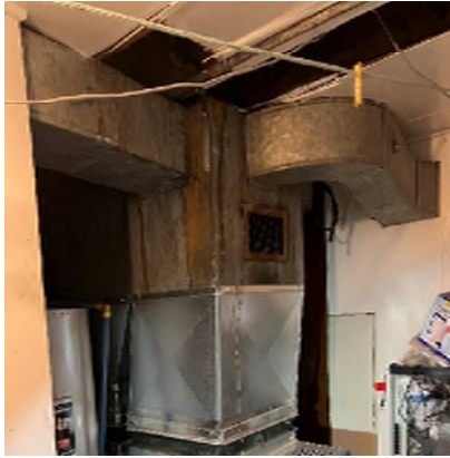
Figure 1-25. Staining on the Ducting Indicating Past Leaks.
