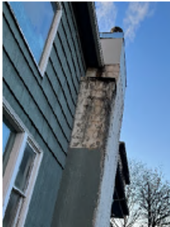
Figure 7-15. Water-Stained Chimney With Visible Cracks.
