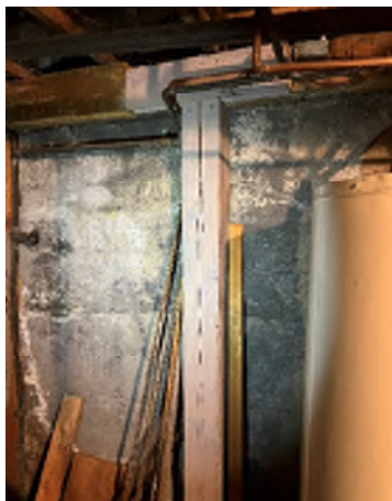
Figure 3-39. Significant Checking in this Column.
