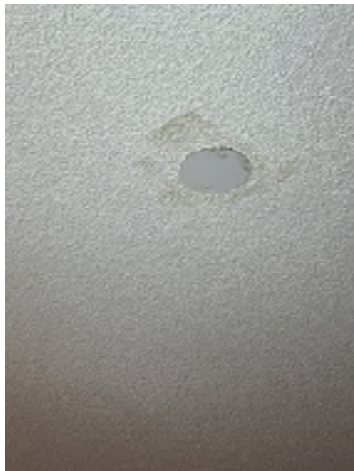
Figure 5-27. Water Damage Around Light Wiring Cover.
