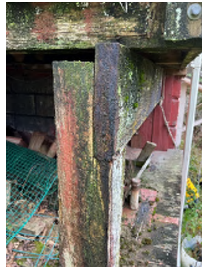
Figure 5-12. Rotten Beam Support and Deck.
