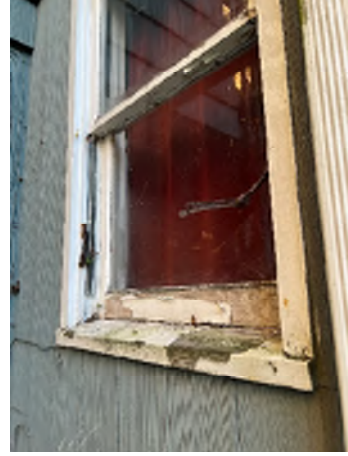
Figure 7-20. Rot at the Windowsill.
