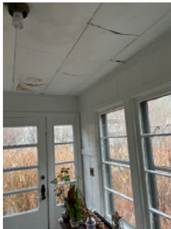
Figure 4-21. Sagging Ceiling and Signs of Water Damage in the East Entryway.
