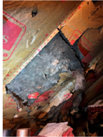
Figure 7-38. Paper Came off the Insulation, and the Insulation Corners Are Falling in the Attic Space.
