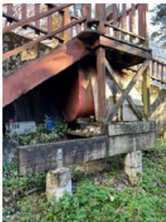
Figure 1-17. Fuel Tank Wedged in the Space Under the stairs.
