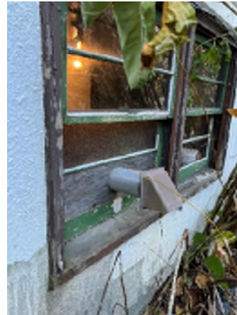
Figure 1-8. Rotten Window Sill.
