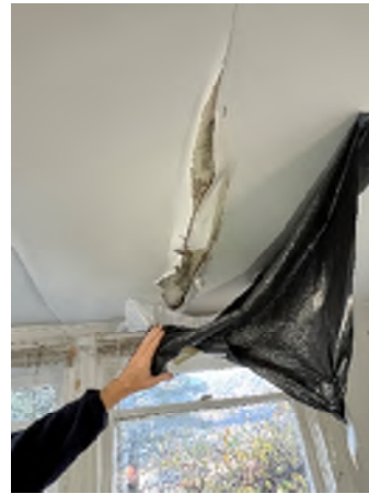
Figure 3-32. More Damage From a Roof Leak Under the Bag.
