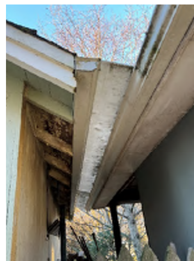
Figure 5-18. Deterioration Under the Eave.
