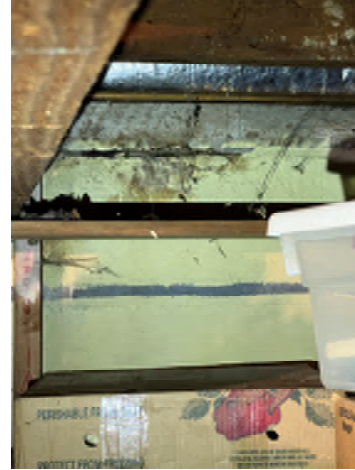
Figure 5-32. Large Crack on the Interior of the Concrete Basement Wall.
