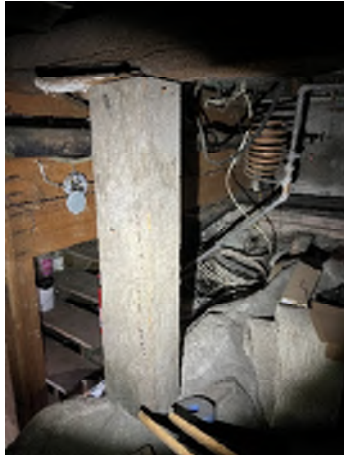
Figure 7-48. One Column Is Sitting on the Bedrock With No Connections. There are shims at the top of the column.
