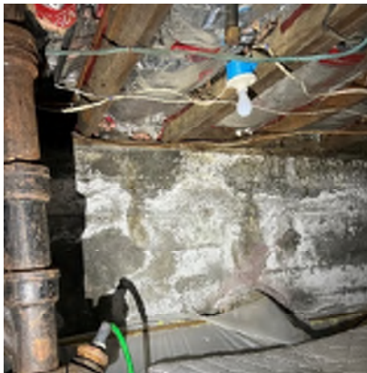
Figure 1-27. Many Signs of Water Infiltration Exist on this Concrete Wall From the Discoloration. The sill plate is rotten from the outside.
