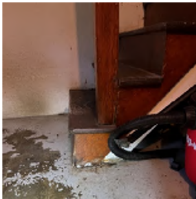
Figure 1-29. Wood at the Bottom of the Stairs Has Some Water Damage.
