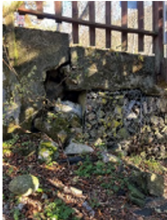
Figure 1-19. Undermining of the Road at the Interface Between the Two Retaining Wall Systems.
