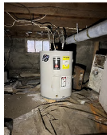
Figure 7-53. The Tank Is Not Seismically Secured.
