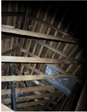
Figure 2-13. Attic Trusses and Most of the Wood Appears Dry. The roof rafters and site built trusses are under sized for current snow loads.
