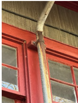
Figure 6-11. Drainpipe Is Rusted.
