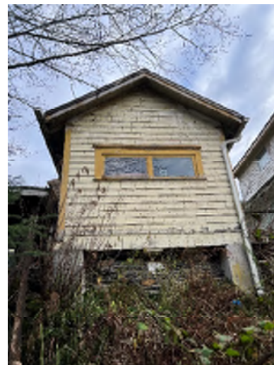
Figure 5-16. West Side of Garage. Paint on the siding has significantly deteriorated.
