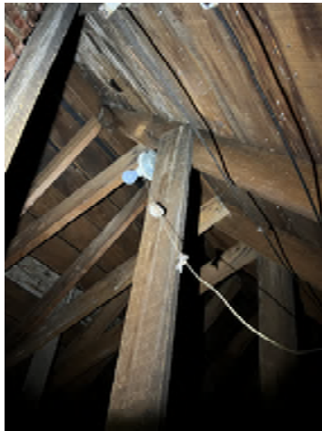
Figure 5-19. Indications of Water Damage on the Roof Rafters.
