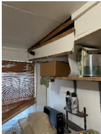
Figure 2-27. Wall Finishes Have Detached.
