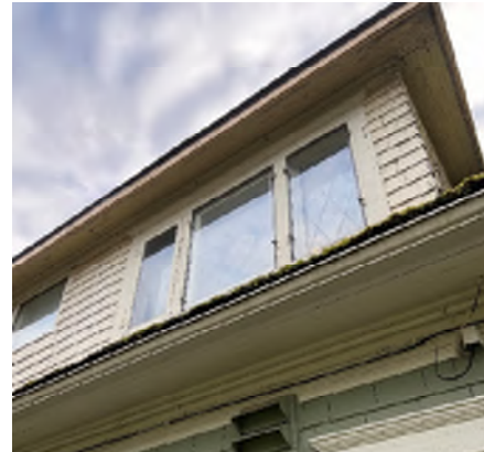
Figure 5-14. Moss on the Roof and Peeling Paint on the Eave.
