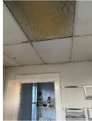
Figure 2-24. Sagging Ceiling Panel in the Kitchen From Water Damage.
