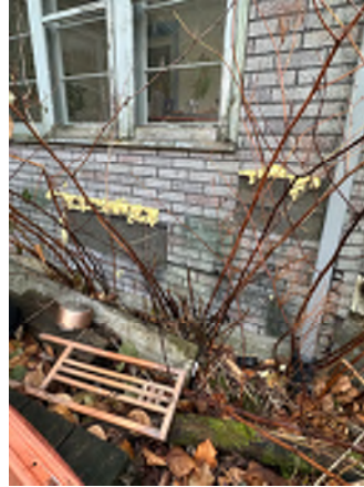
Figure 4-4. Siding Replaced With Roof Shingles and Spray Foam.
