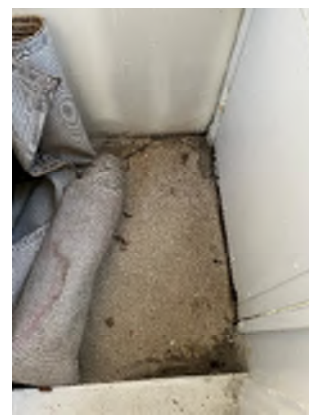
Figure 7-30. Moisture Damage and Rot in the Back Entryway.
