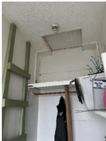
Figure 2-19. Inadequate Framing to Support the Closet Used for Attic Access.
