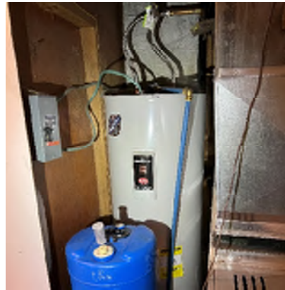
Figure 1-26. Water Heater Without Seismic Strapping.
