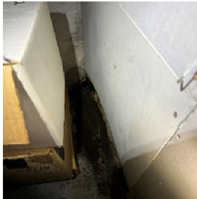
Figure 1-30. Channel Under the Stairs Where Water Frequently Flows In. This is the location of the large concrete crack on the north side wall.
