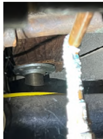
Figure 2-38. A Pipe Supporting a Beam With No Positive Connections at the Top or Base.
