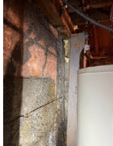
Figure 3-38. No Positive Connection From this Column to the Beam Above and the Column Has Shifted.
