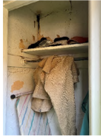
Figure 3-20. Significant Sheetrock Damage in the Closet.
