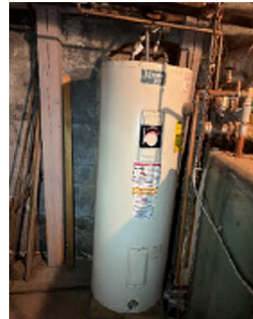
Figure 3-40. No Seismic Strapping Around the Water Heater.
