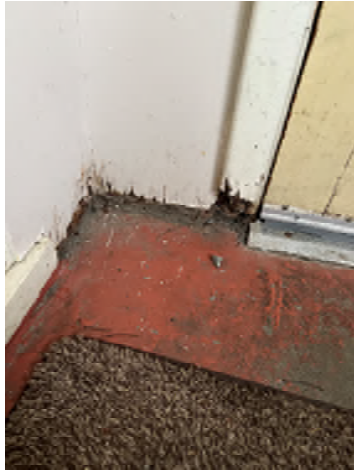
Figure 5-25. Rotting Wood Next to the Entryway Door.
