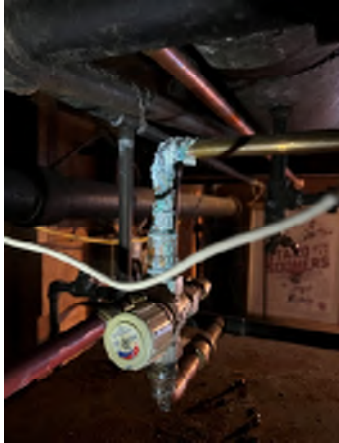
Figure 2-35. Signs of Leaks and Corrosion Exist at the Pipe Connections.
