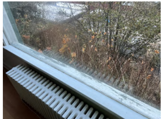
Figure 7-42. The Window Frame Has Some Deterioration.
