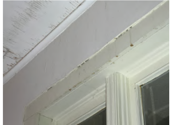
Figure 5-26. Indications of Water Damage on Windowsill.
