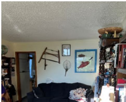
Figure 1-21. Very Few Sheetrock Cracks Were Observed on the Main Level.
