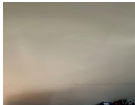
Figure 1-24. The Only Cracks Observed Were at the Sheetrock Panel Joints.
