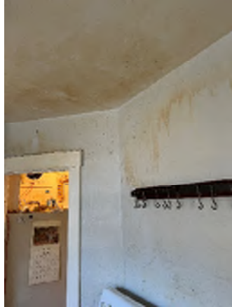
Figure 3-25. A Significant Amount of Discoloration on the Sheetrock Above the Stove in the Kitchen, Water Damage.
