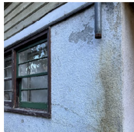
Figure 1-6. The Drainpipe Ends Abruptly in Mid-Air and Does Not Direct Water Away From the Foundation.
