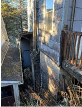
Figure 3-13. South Side of the Building and Rotten Deck.
