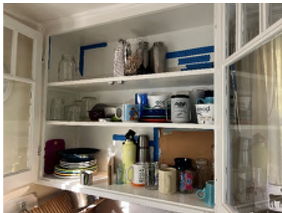
Figure 3-35. Blue Tape Where the Tenant Found Cracks.
