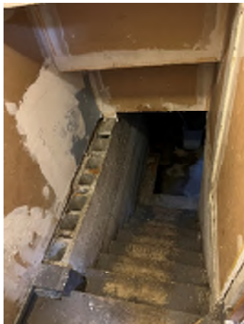
Figure 7-45. No Grout Columns Were Observed in the Visible Portion of the Masonry Wall. This wall is likely unreinforced.
