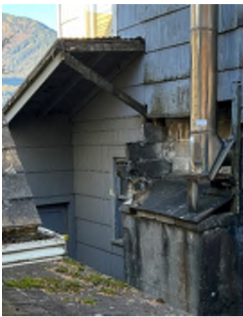
Figure 3-18. Concrete Blocks Not Adequately Secured. The new stack is partially supported on a rotten piece of plywood.
