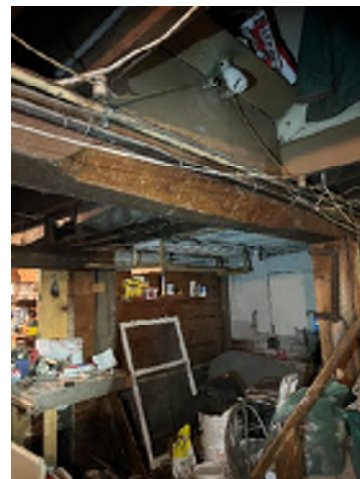
Figure 3-42. Notched Large Beam at the Bottom of the Stairs to prevent head injury.
