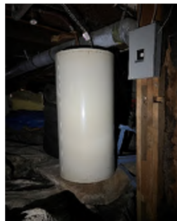
Figure 7-52. The Tank Is Not Seismically Secured.
