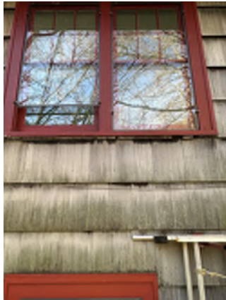
Figure 6-9. Deteriorating Window Sill.
