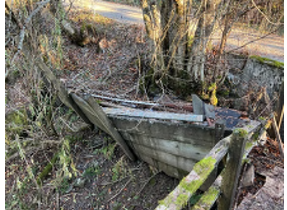
Figure 3-8. Failed Wooden Retaining Wall.
