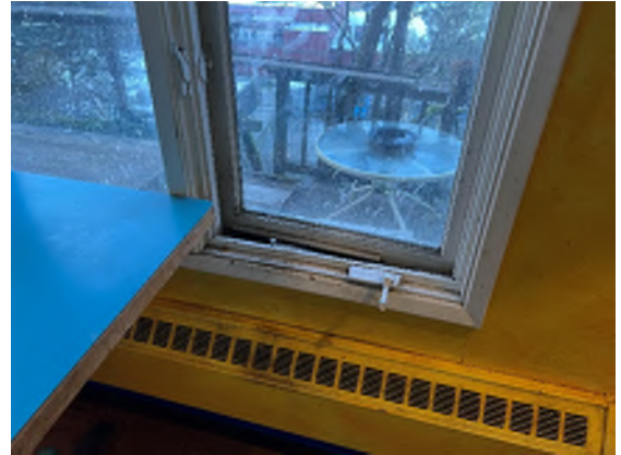
Figure 7-44. One Window No Longer Opens Properly.
