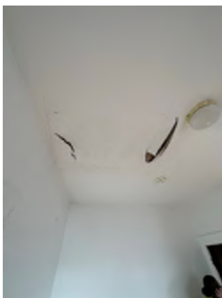
Figure 4-29. Peeled Paint and Cracked Sheetrock on the Ceiling from Water Damage.
