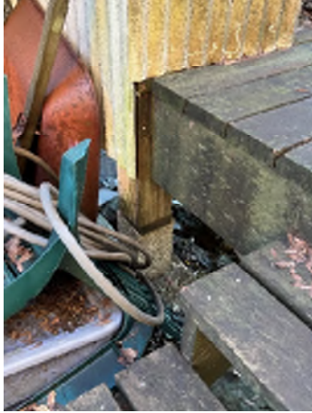
Figure 7-19. Moss Growing on the Deck. The column is shimmed and sitting on a concrete pile.
