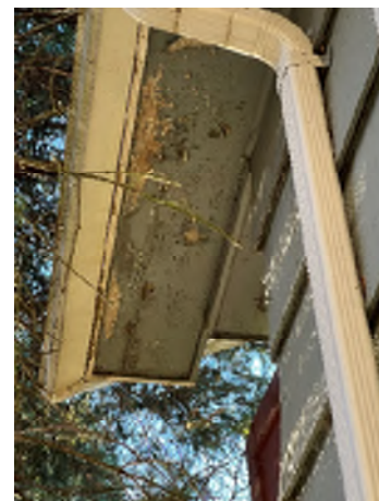
Figure 7-24. Deterioration to the Underside of the Eave.
