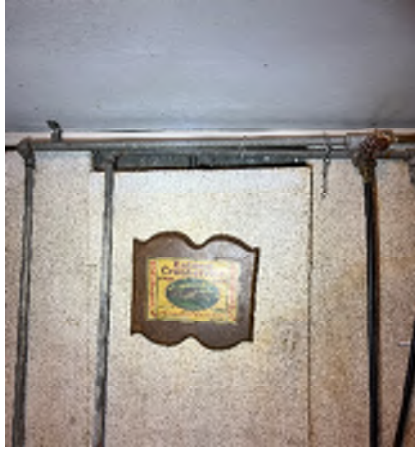
Figure 2-29. Wall Panel Has Detached From the Wall.
