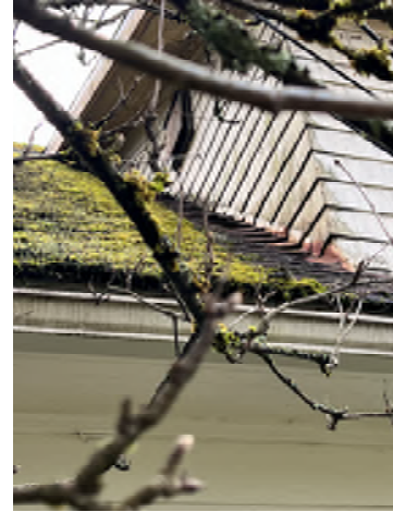
Figure 5-2. Moss on the Roof and Deteriorating Shingles and Siding.
