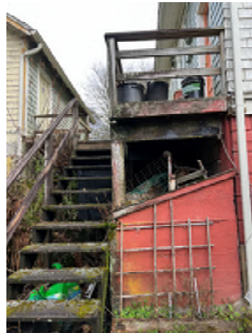
Figure 5-10. Rotted Deck and Stairs. Deck posts are not anchored and have no positive connection to joists.
