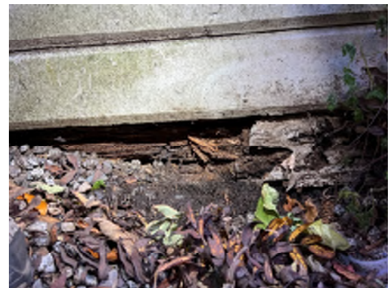
Figure 1-16. Exposed Wood Beneath the Siding Is Rotten.
