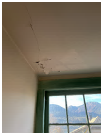
Figure 6-17. Cracking and Peeling Paint on the Ceiling.
