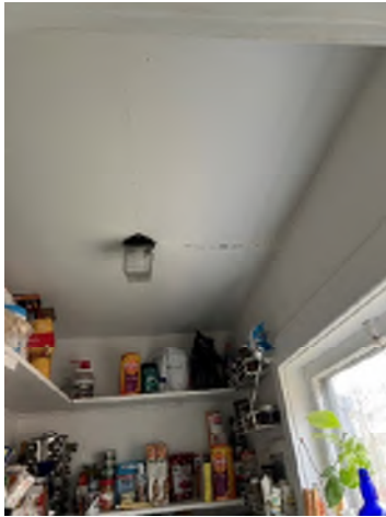
Figure 4-25. Sheetrock Cracks at Panel Edges.
