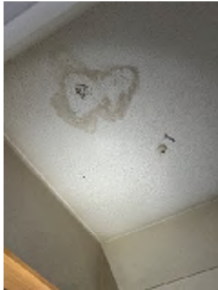
Figure 2-23. Water Damage, Cracks, and Exposed Wiring in the Closet on the Northeast Side of the Building.
