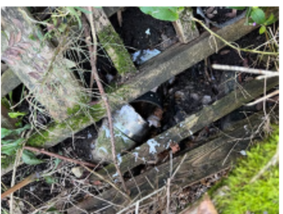
Figure 7-12. A Broken Pipe Below the Pile of Wood That May Be a Sewer Pipe.
