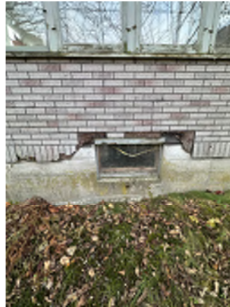
Figure 4-6. Deteriorated Siding and Windowsills.
