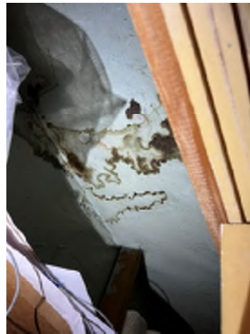
Figure 4-26. Staining on Ceiling.
