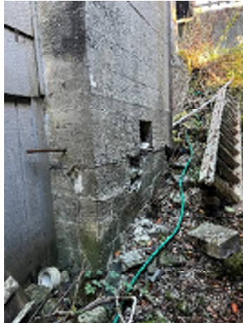
Figure 3-15. Failed Chimney Foundation Wall. Collapse Hazard.
