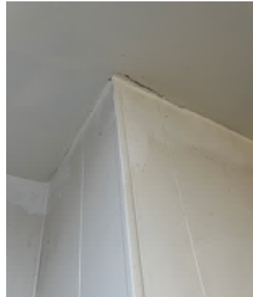
Figure 5-24. Continuous Ceiling Crack Around a Corner.
