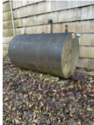
Figure 6-8. Fuel Tank Is Not Seismically Anchored.
