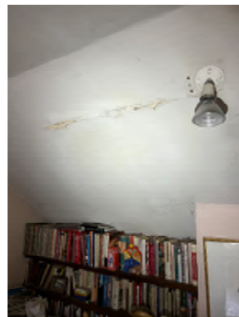
Figure 6-18. Cracking and Indications of Water Damage on the Ceiling.
