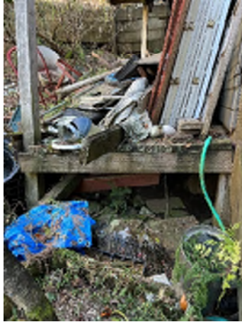
Figure 3-7. Moss and Rot on the Deck.
