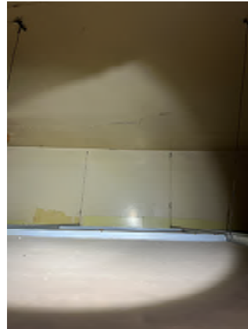
Figure 5-28. Cracks in the Ceiling Above the Dropped Ceiling in the Kitchen.
