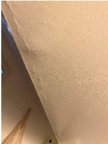
Figure 7-37. Paint Is Chipped, and the Sheetrock Fasteners Are Visible in Some Places.
