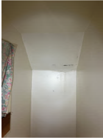
Figure 6-19. Cracking and Water Damage Indications Above the Stairs.
