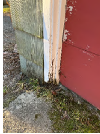
Figure 7-26. Rot Near the Ground.
