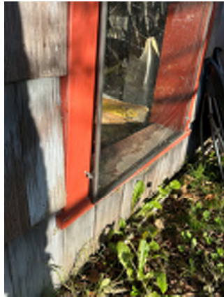
Figure 6-13. Gap in the Storm Window.
