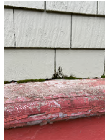
Figure 5-4. Deteriorated Siding With Moss Growing in the Gaps.
