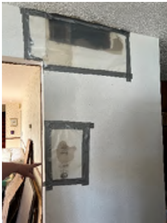
Figure 7-33. Damage to the Finishes Caused by the Sink Leak.
