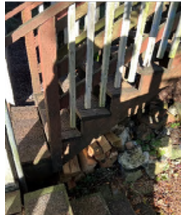
Figure 1-20. A Long Crack on the Side of the Stringer.
