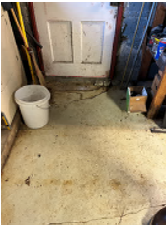
Figure 6-22. Cracked Slab-on-Grade at the North Basement Entrance.
