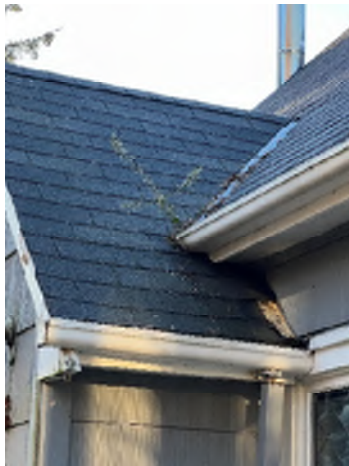
Figure 3-3. Plant Growth indicates Build-up in Gutter.
