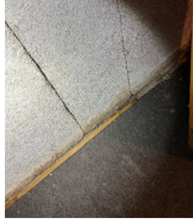
Figure 2-30. Bottom of the Wall Panel Has Water Damage.
