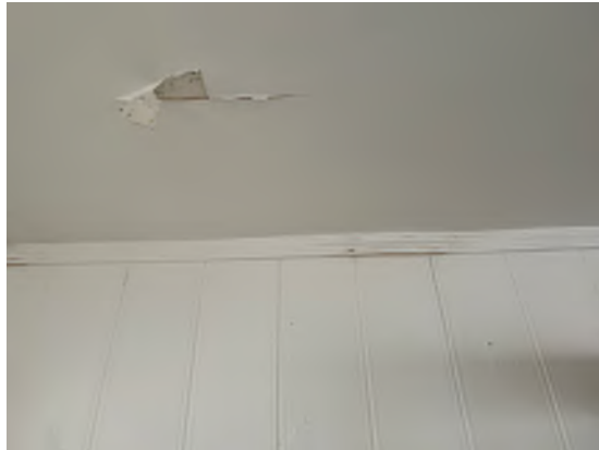
Figure 4-19. Peeled Paint With Signs of Water Damage on the Ceiling and Cracking in the Trim and Wallboards.
