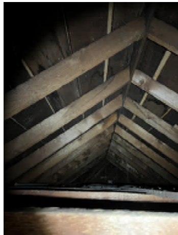
Figure 6-15. Signs of Old Water Damage. New roof sheathing exists above the old boards that appears to be in good condition.
