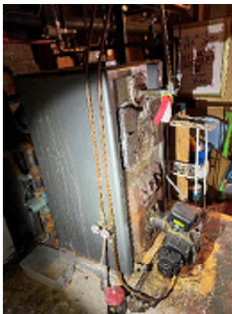
Figure 2-33. Signs of Leaks Exist With the Staining on the Side of the Unit.
