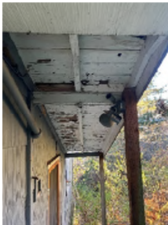
Figure 3-9. Peeling Paint and Fixtures Missing Bulbs; Open Fixtures or Exposed Wiring Can Be Hazardous.
