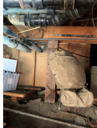
Figure 6-25. No Lateral Restraint/Connection From Beam to Column. The wood column is placed directly on top of the rock.
