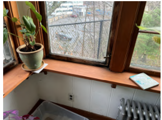
Figure 4-20. Rotting Window Frame.
