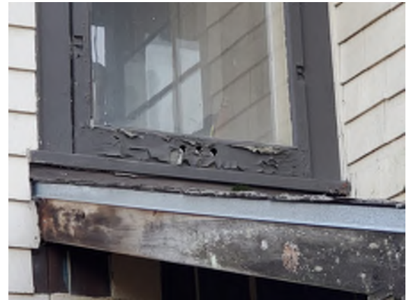
Figure 2-2. Three Holes in the Window That Could Allow Water to Enter the Building.
