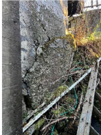
Figure 3-16. Cracked Concrete Wall/ Failed Foundation, Possibly From Flexure and Shifting. No reinforcement was observed. Collapse Hazard.
