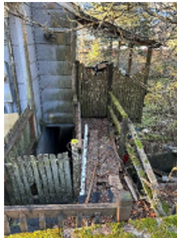
Figure 3-4. Rotten Gates, Railings, and Deck Framing Pose a Safety Hazard and Should Not Be Used.
