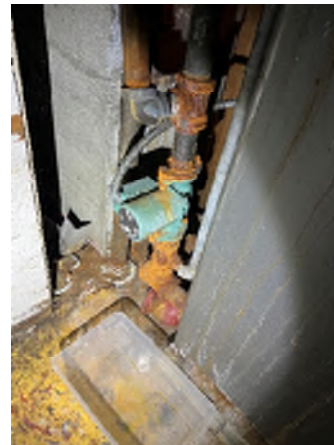
Figure 2-34. Signs of Leaks Exist at the Pipe Connections.
