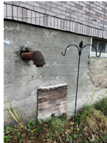
Figure 4-10. Large Hole Where Pipe Exits the Basement and Cracking Between the Different Concrete Pours Under Window.
