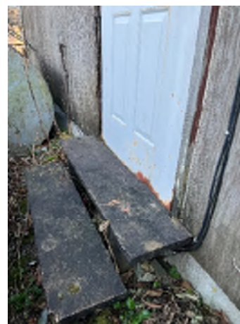
Figure 7-6. Unprotected Plywood Sheathing by the Siding and Rust Around the Man Door.
