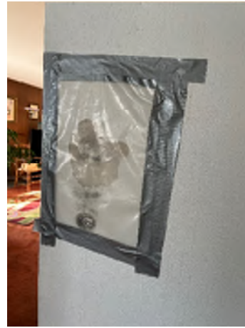
Figure 7-34. Mold Is Growing Under the Vapor Barrier. The Extent of Damage in the Wall Cavity Is Unknown.
