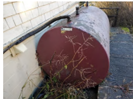
Figure 2-12. Tank Is Not Seismically Anchored.
