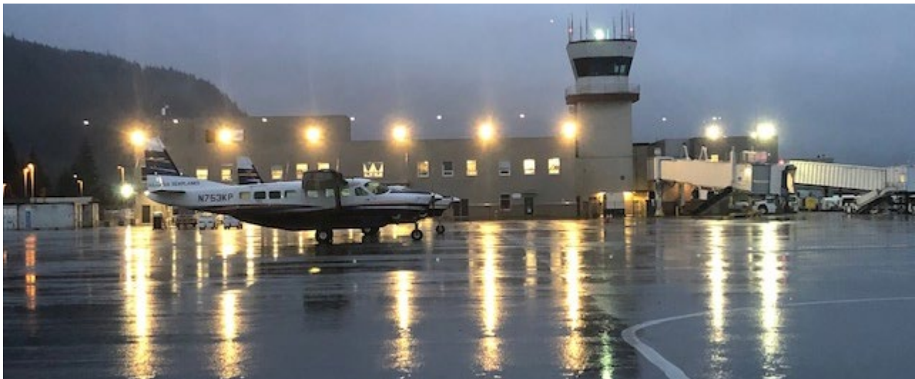
PHOTO 01: The six new LED ramp lighting fixtures are shown on the left-center of the photo. The two old fixtures are shown on the right.
