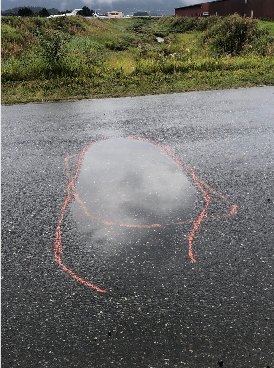
Photo 03: Extent of depression in the asphalt paving directly above the culvert.
