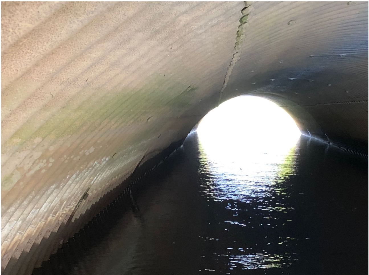
Photo 02: Visible deformation in the north wall of the culvert.
