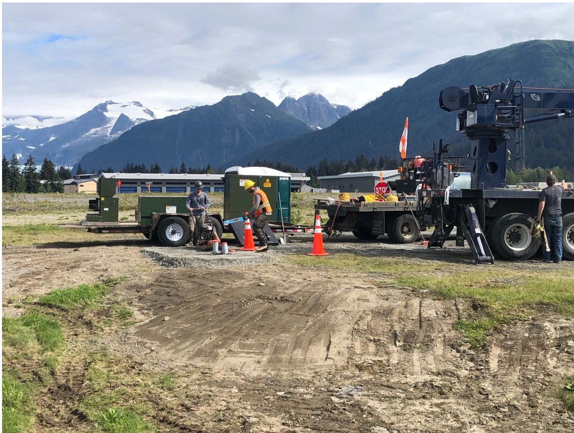
Photo 01: AEL&P preparing the transformer pad near the west end of the float pond.
