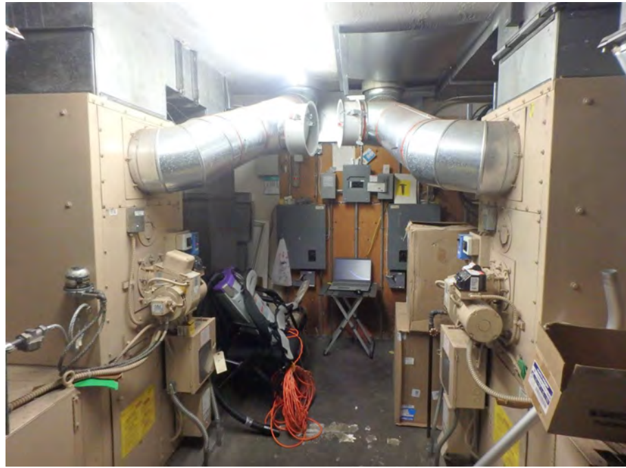
2 nd floor mechanical room
