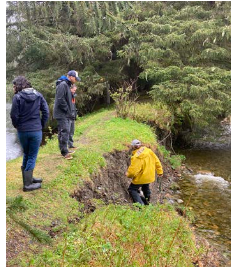
A section of dike between Fish Creek (right) and the Northeast Pond (left) that is experiencing severe erosion.
