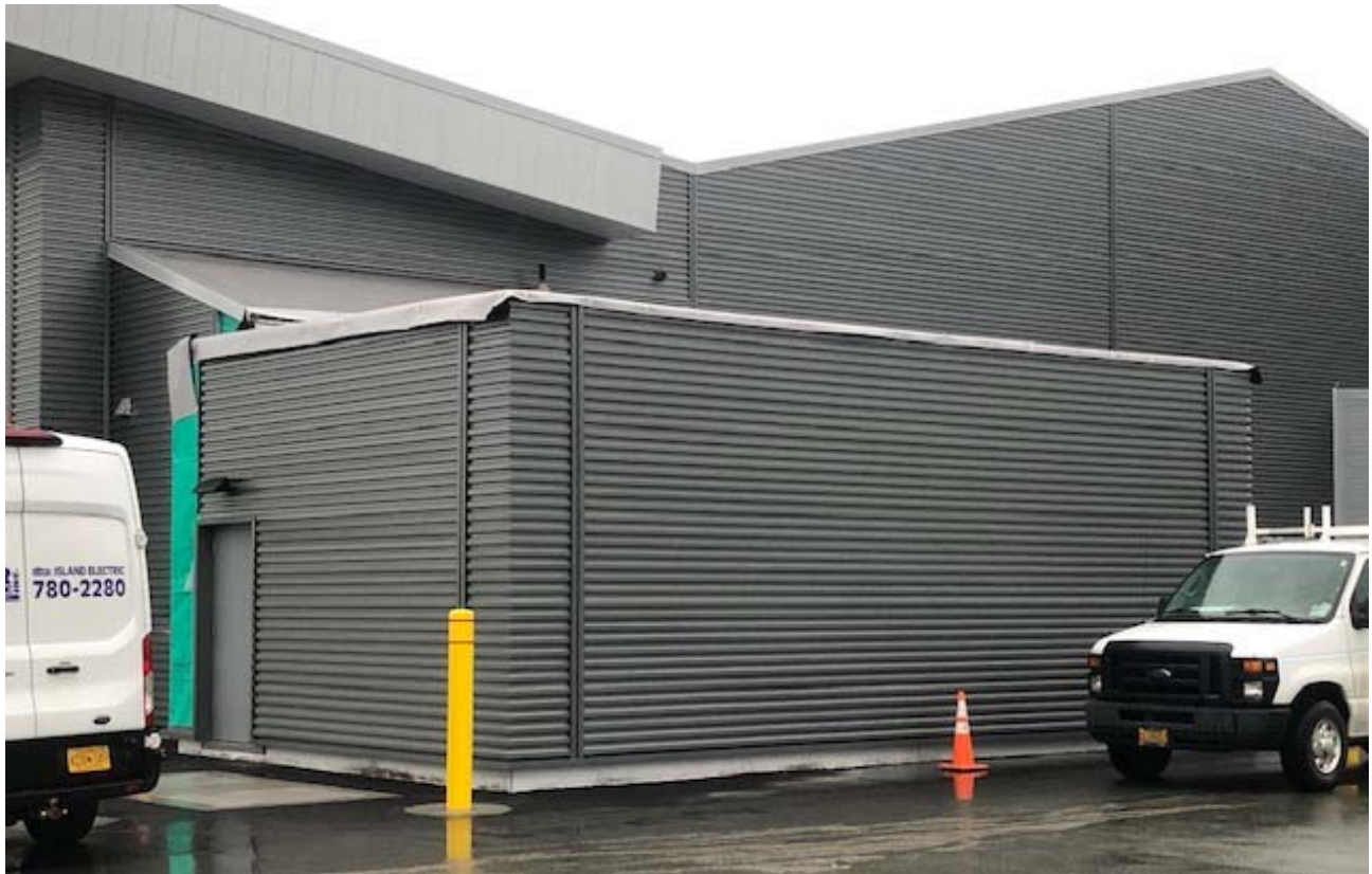
Photo 05: Exterior metal siding work nearly complete on the new ALRV addition to the SREB.
