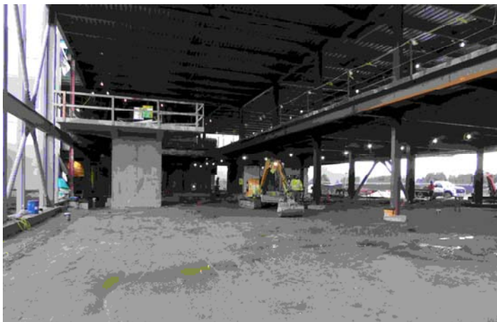
Looking south toward open stair, with balcony outside of airport administration office on upper level.
