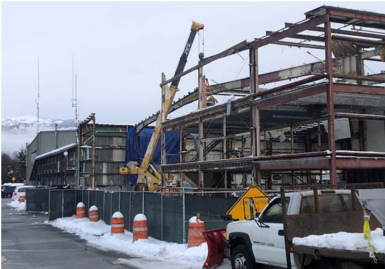
Figure 1-1: Removal of the secondary steel from the roof of the old Sand Shed.
