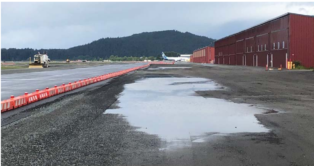
Figure 1 - Ponding in existing RAP apron located on the south side of the Block O hangars.
