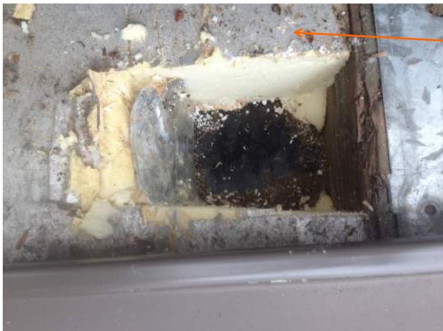
NO BARRIER MEMBRANE - MOISTURE WHICH PENETRATES METAL ROOF PANEL ASSEMBLY ENTERS DIRECTLY INTO INSULATION CAVITY AND STRUCTURE BELOW
