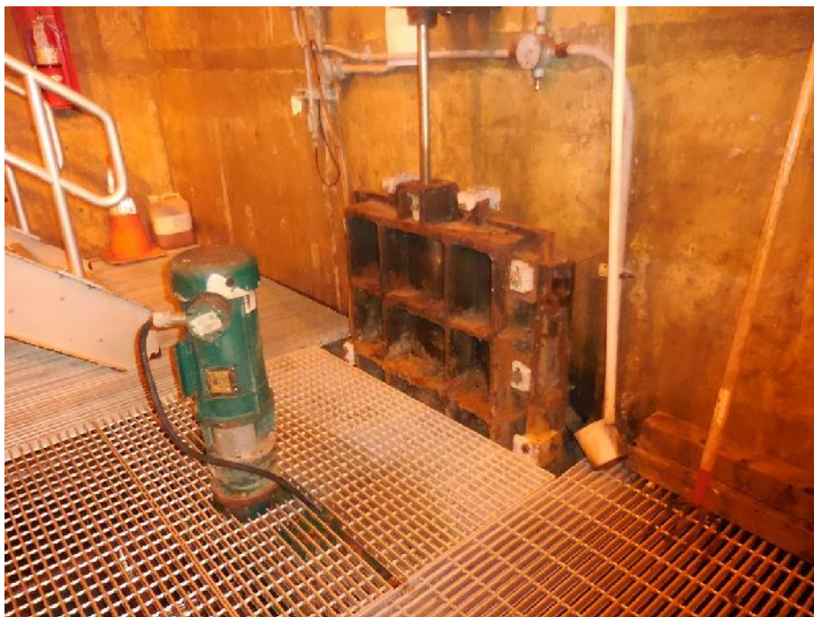
Figure 3. Influent Gate Valve
