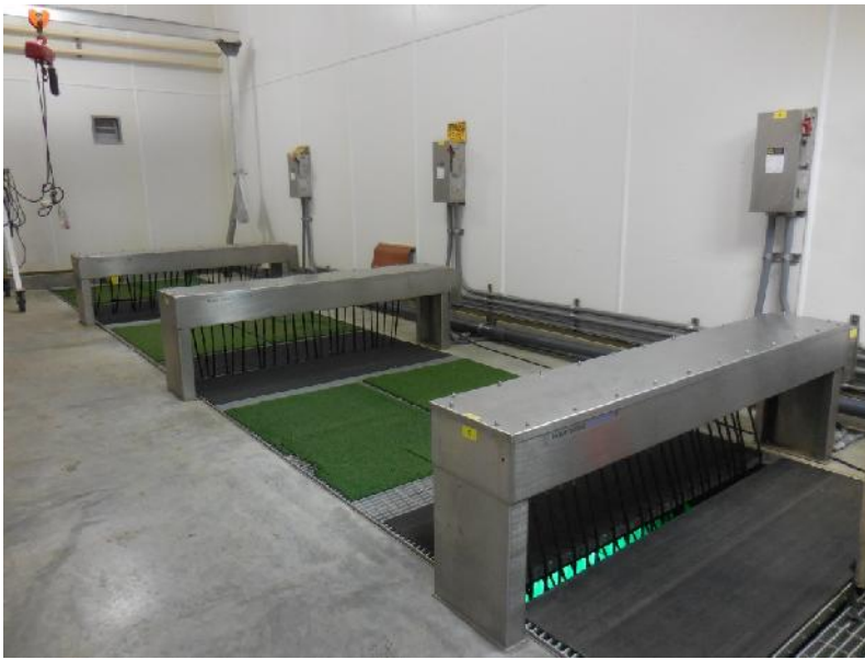
Figure 10. UV Disinfection System
