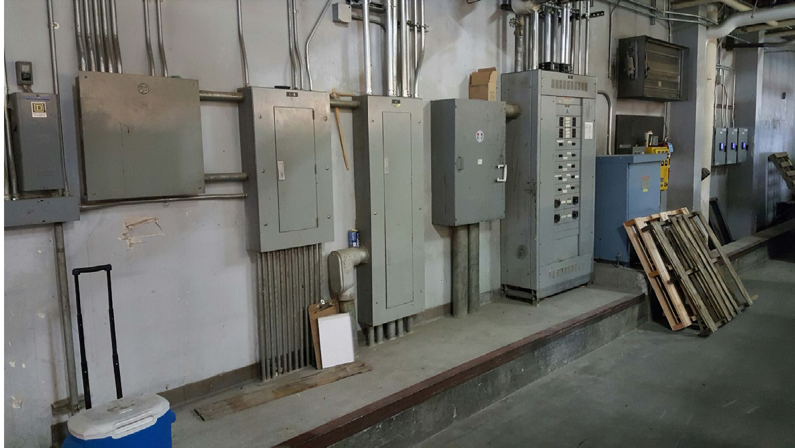
1 PHOTO - EXISTING PANEL BOARDS
