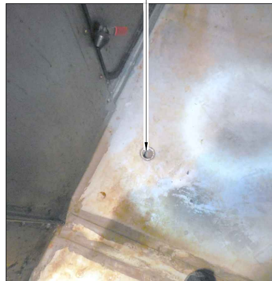
4 EXHIBIT PHOTO - COMPARTMENT #8 MIXED AIR DISCHARGE
