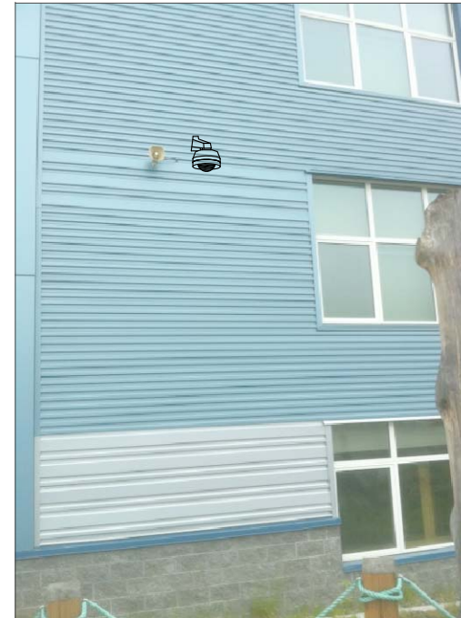
CHB7- WALL MOUNT. BACK FEED TO ABOVE CEILING IN CLASSROOM, THEN TO SWITCH IN IT ROOM.
