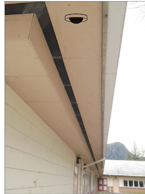
CR8- CEILING MOUNT IN SOFFIT, FEED FROM ABOVE SUSPENDED CEILING. THEN ROUTE IN WIREMOLD 500 RACEWAY DOWN TO EXISTING RACEWAY. THEN VIA EXISTING RACEWAY TO IT CABINET.
