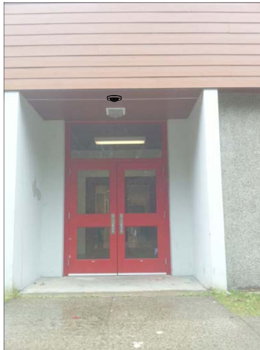
CF8- FEED FROM ABOVE SUSPENDED CEILING IN HALL THROUGH SOFFIT SPACE TO CAMERA..
