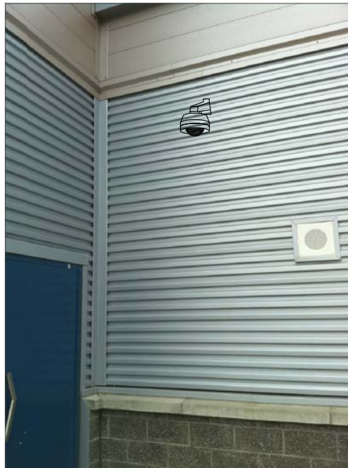
CT17- WALL MOUNT, FEED FROM ABOVE CEILING IN LOCKER ROOM TO HALLWAY CEILING, THEN ABOVE HALLWAY CEILING TO IT CABINET.
