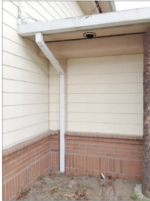
CR1- CEILING MOUNT, FEED THROUGH SOFFIT TO WIREMOLD J-BOX, THEN IN WIREMOLD 500 DOWN INTERIOR OF WALL TO EXISTING SURFACE RACEWAY, THEN VIA RACEWAY TO IT CABINET.
