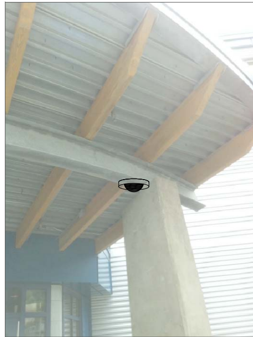
CHB2- SURFACE MOUNT TO INSIDE OF BEAM. SURFACE MOUNT CONDUIT TO METAL FASCIA INSIDE FASCIA PANELS ABOVE CEILING IN ADMINISTRATION BUILDING.
