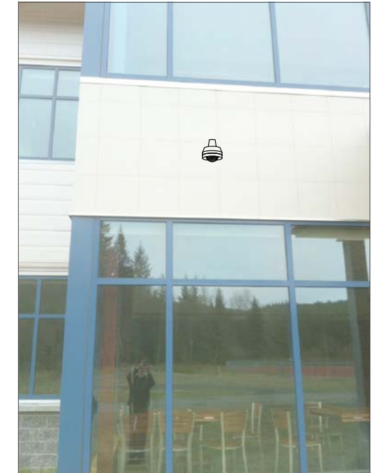
CT8- WALL MOUNT, FEED FROM ABOVE INTERIOR SUSPENDED CEILING. ROUTE ABOVE SUSPENDED CEILING TO IT CABINET.
