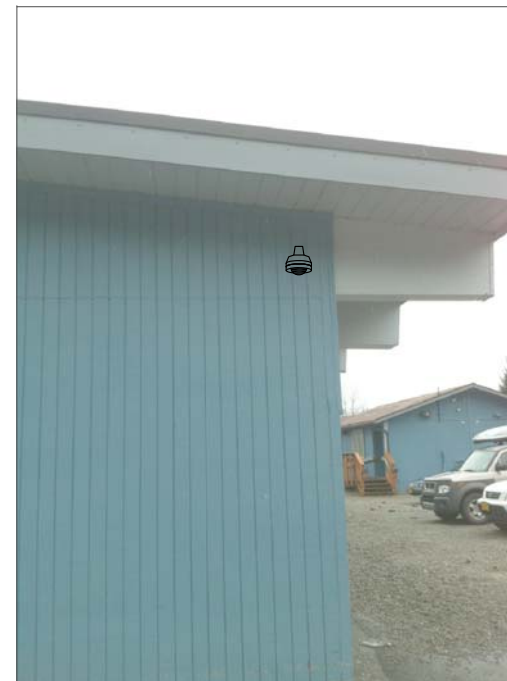
CG10a- WALL MOUNT UNDER EAVE, FEED FROM IT CABINET WITH SURFACE WIREMOLD UP WALL INSIDE CLASSROOM.
