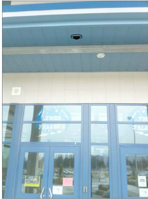
CT1- CEILING MOUNT, FEED FROM ABOVE SOFFIT METAL. SURFACE MOUNT CONDUIT IN ENTRY TO WALL/CEILING. ROUTE TO NEAREST SUSPENDED CEILING, THEN ABOVE SUSPENDED CEILING TO IT CABINET.
