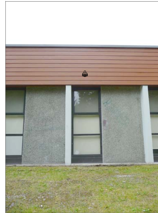
CF7d- WALL MOUNT TO HARDI PLANK, FEED FROM ABOVE SUSPENDED CEILING IN CLASSROOM, AIM AT BREAK IN FENCE. SUSPENDED CEILING AT 9'-10".
