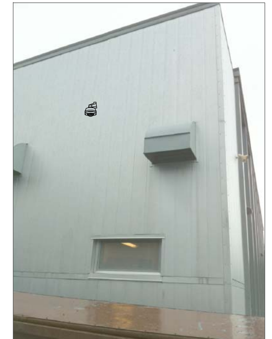
CG14- MOUNT ABOVE AND BETWEEN TWO DUCTS. THE DUCTS FEED FROM EXISTING SURFACE RACEWAY IN GYM. (5)
