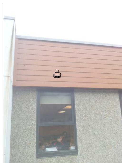
CF5- WALL MOUNT TO HARDI PLANK. FEED FROM ABOVE SUSPENDED CEILING IN CLASSROOM. SUSPENDED CEILING AT 9'-10".
