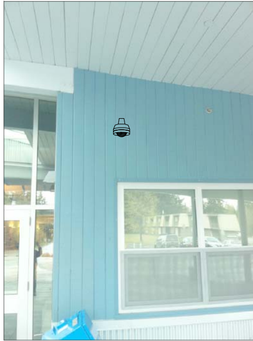
CG1- MOUNT TO WALL ABOVE SUSPENDED CEILING. FEED FROM ABOVE CEILING IN OFFICE. SUSPENDED CEILING AT 9'.
