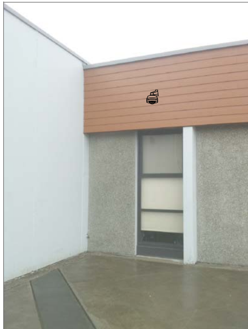
CF2- WALL MOUNT TO HARDI PLANK. FEED FROM ABOVE SUSPENDED CEILING IN CLASSROOM. SUSPENDED CEILING AT 9'-10".
