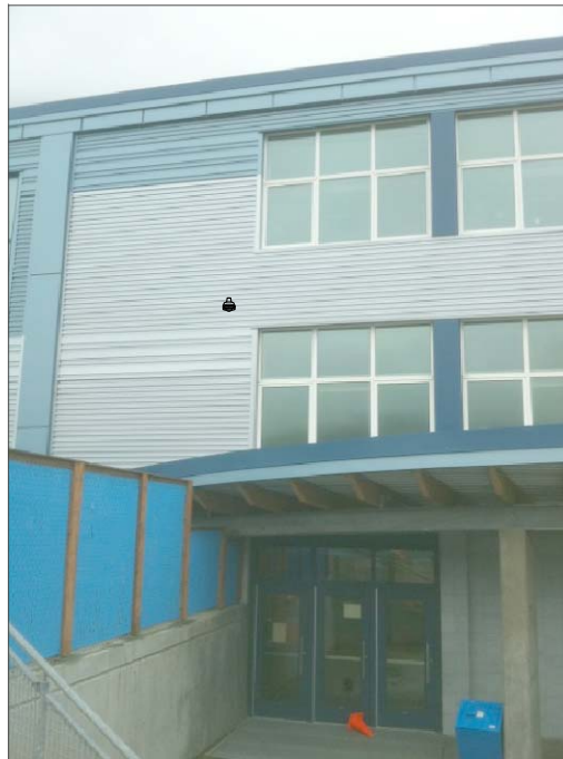
CHB9- WALL MOUNT. BACK FEED TO ABOVE CEILING IN CLASSROOM, THEN TO SWITCH IN IT ROOM.
