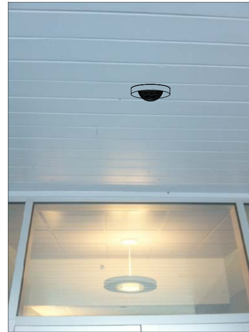
CG3- CEILING MOUNT, FEED FROM ABOVE SUSPENDED CEILING IN HALL. SUSPENDED CEILING AT 9'
