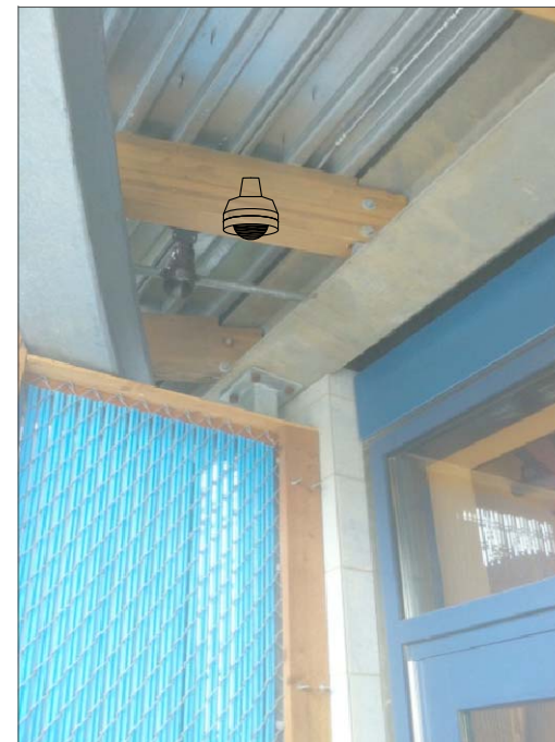
CHB10a- WALL MOUNT ON GLUELAM. FEED SURFACE UNDER STEEL BEAM AND INTO LUNCHROOM ON CEILING THEN ABOVE SUSPENDED CEILING IN HALL AND INTO THE SWITCH IN THE IT CABINET.
