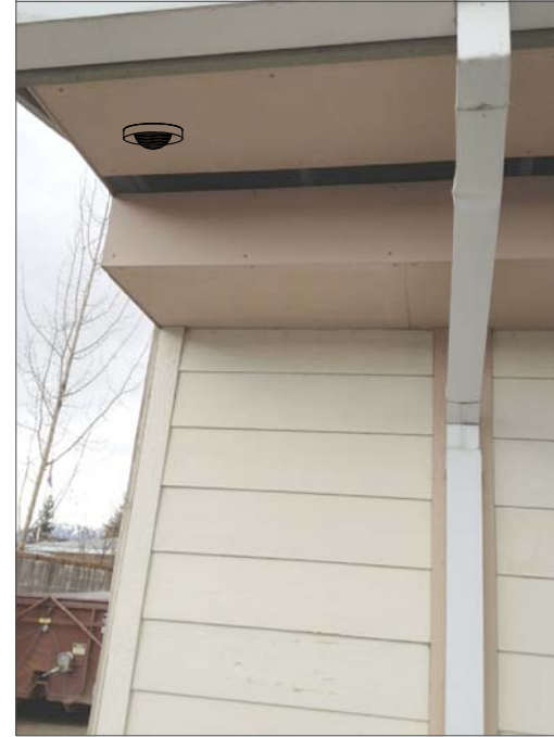
CR15- CEILING MOUNT, FEED THROUGH SOFFIT. SURFACE MOUNT CONDUIT IN MECHANICAL SPACES TO IT CABINET ON SECOND FLOOR. (4)
