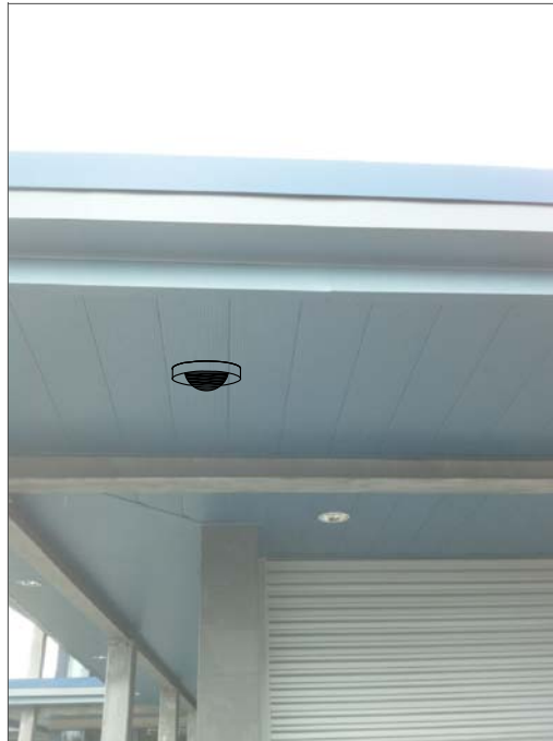
CT18- CEILING MOUNT, FEED FROM ABOVE CEILING IN WEIGHT ROOM, THEN ABOVE HALLWAY CEILING TO IT CABINET.
