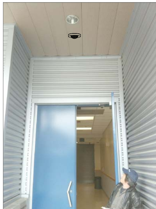
CT14- CEILING MOUNT, FEED FROM ABOVE CORRIDOR CEILING. ROUTE ABOVE SUSPENDED CEILING TO IT CABINET.
