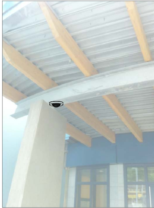
CHB1- SURFACE MOUNT TO INSIDE OF BEAM. SURFACE MOUNT CONDUIT TO METAL FASCIA INSIDE FASCIA PANELS ABOVE CEILING IN ADMINISTRATION BUILDING. (5)
