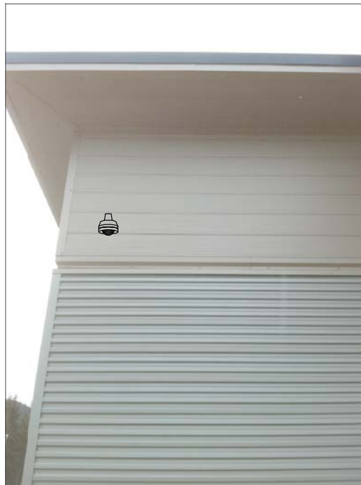
CT13- EXTERIOR MOUNT ABOVE SUSPENDED CEILING IN CHOIR ROOM, FEED FROM ABOVE INTERIOR CEILING. ROUTE ABOVE SUSPENDED CEILING TO IT CABINET.
