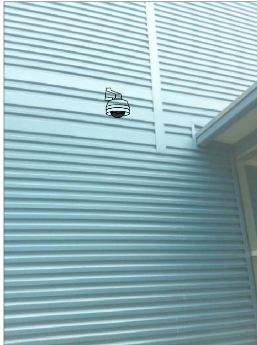
CHB5- WALL MOUNT. BACK FEED TO ABOVE CEILING IN CLASSROOM, THEN TO SWITCH IN IT ROOM.
