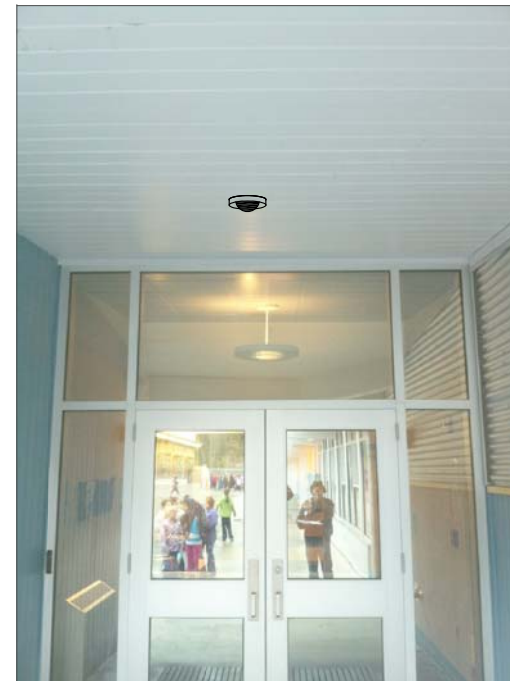
CG7- CEILING MOUNT FEED FROM ABOVE SUSPENDED CEILING IN HALL. SUSPENDED CEILING AT 9'.
