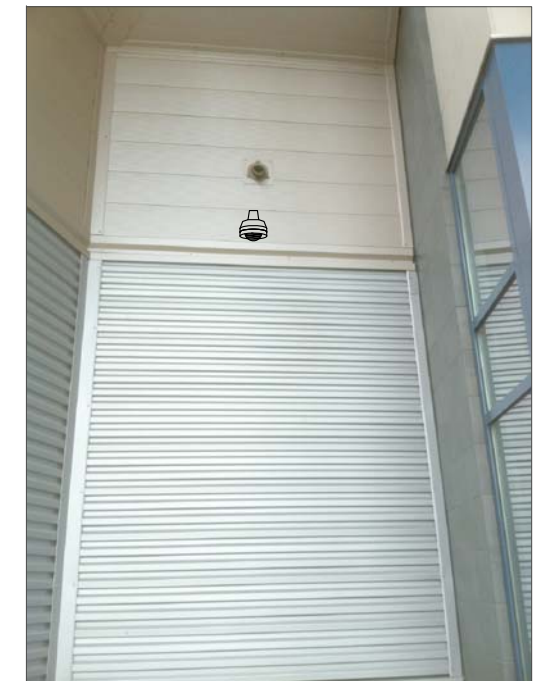
CT12- EXTERIOR WALL MOUNT ABOVE INTERIOR CEILING, FEED FROM ABOVE CEILING. ROUTE ABOVE SUSPENDED CEILING TO IT CABINET.
