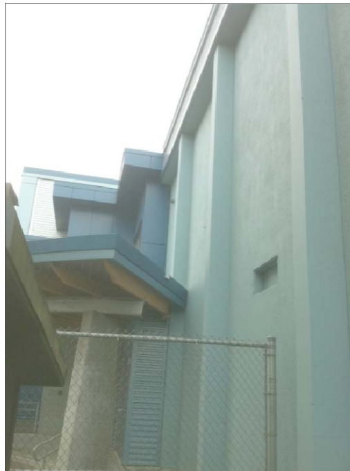
CHB11- ROUTING ON BUILDING EXTERIOR UP WALL IN CORNER TO UNDER EAVE, THEN BELOW EAVE TO OPPOSITE ENTRY CEILING. THEN TO ABOVE CLASSROOM 206 CEILING.
