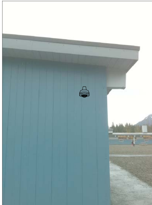
CG5- WALL MOUNT, FEED WITH SURFACE WIRE MOLD UP INSIDE WALL FROM EXISTING SURFACE RACEWAY IN CLASSROOM.
