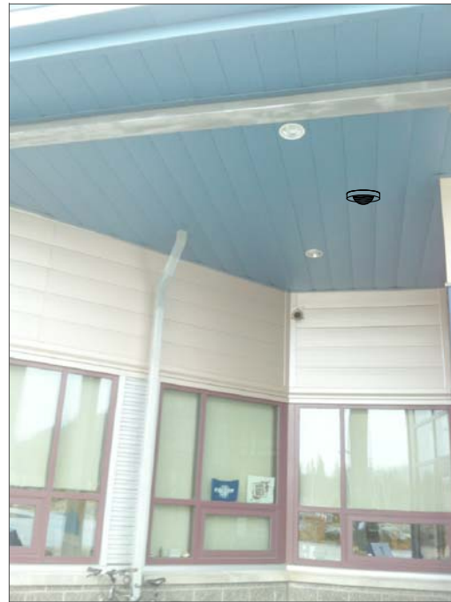
CT2- CEILING MOUNT, FEED FROM ABOVE SOFFIT METAL INTO SPACE ABOVE SUSPENDED CEILING, THEN ABOVE SUSPENDED CEILING TO IT CABINET.
