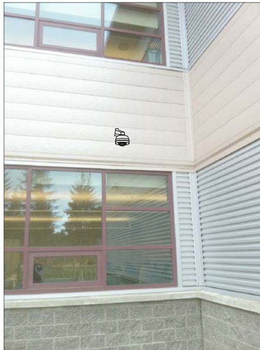
CT9- WALL MOUNT, FEED FROM SUSPENDED CEILING ABOVE CLASSROOM. ROUTE ABOVE SUSPENDED CEILING TO IT CABINET.
