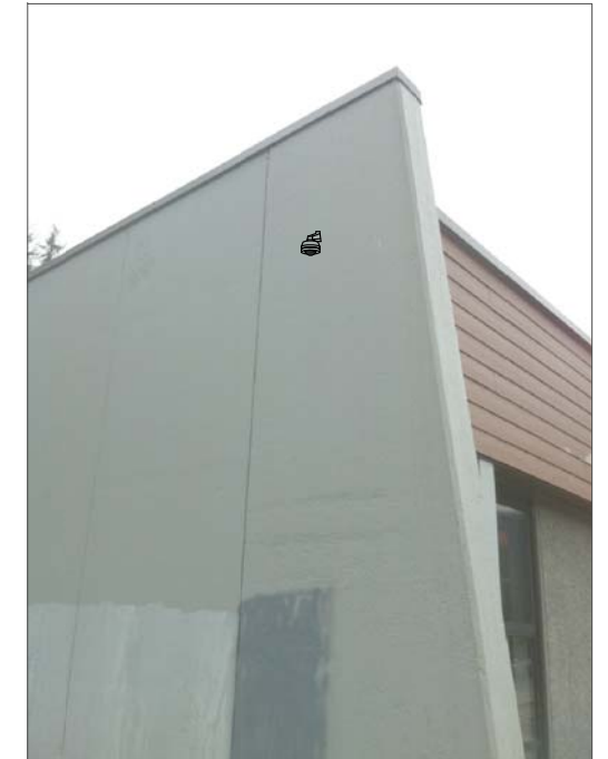
CF11- WALL MOUNT, FEED FROM ABOVE SUSPENDED CEILING THROUGH HARDI PLANK THEN SURFACE UP AND OVER PARAPET THEN DOWN TO CAMERA.
