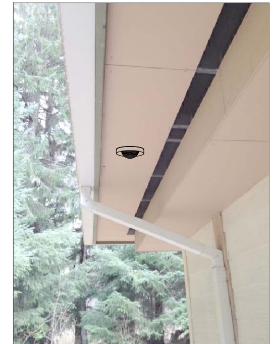
CR6a- CEILING MOUNT IN SOFFIT, FEED FROM ABOVE SUSPENDED CEILING IN CLASSROOM. THEN DOWN CLASSROOM WALL IN WIREMOLD 500 DOWN TO EXISTING RACEWAY THEN VIA EXISTING RACEWAY TO IT CABINET.
