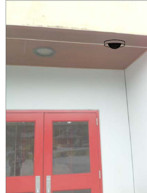
CF4- CEILING MOUNT TO SIDE AND CLOSE TO EDGE OF SOFFIT. FEED FROM ABOVE SUSPENDED CEILING, THROUGH SOFFIT SPACE THEN TO CAMERA.
