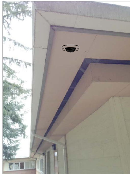
CR7a- CEILING MOUNT IN SOFFIT FEED FROM ABOVE SUSPENDED CEILING IN CLASSROOM. THEN ROUTE IN WIREMOLD 500 RACEWAY DOWN TO EXISTING RACEWAY. THEN VIA EXISTING RACEWAY TO IT CABINET.
