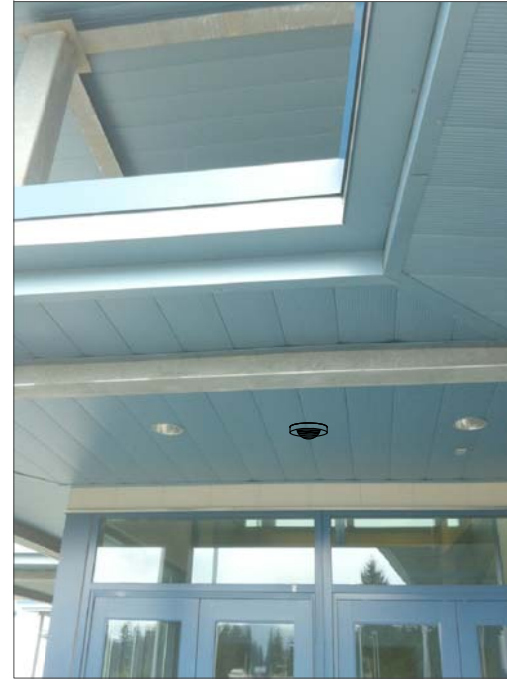
CT19- CEILING MOUNT, FEED FROM ABOVE CEILING IN WEIGHT ROOM, THEN ABOVE HALLWAY CEILING TO IT CABINET.
