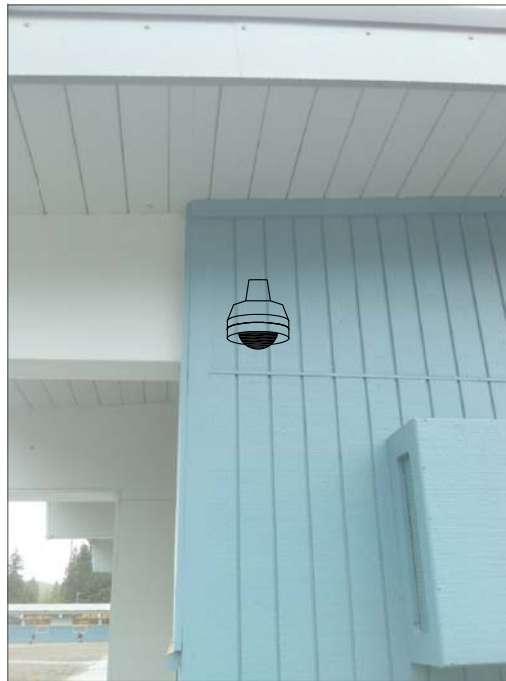
CG9- WALL MOUNT UNDER EAVE, FEED FROM IT CABINET WITH SURFACE WIREMOLD UP WALL INSIDE CLASSROOM. (5)
