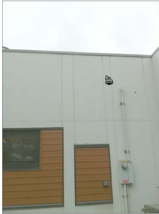
CF7b- WALL MOUNT SAME HEIGHT AS CF7a. FEED FROM ABOVE SUSPENDED CEILING IN CLASSROOM.
