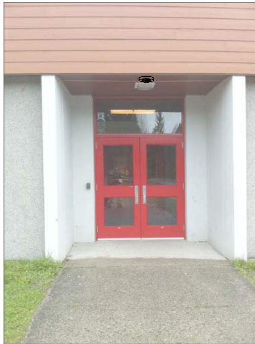
CF12- CEILING MOUNT IN SOFFIT, OUT IN FRONT OF LIGHT. FEED FROM ABOVE SUSPENDED CEILING IN HALL THROUGH SOFFIT SPACE TO CAMERA.
