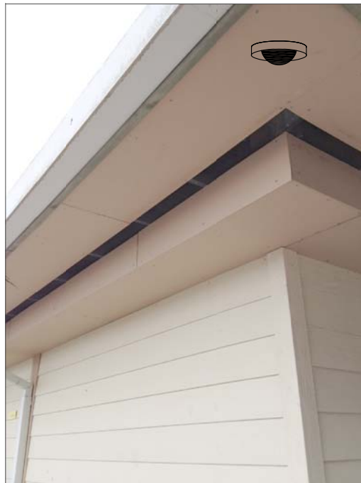
CR9a- CEILING MOUNT IN SOFFIT, FEED FROM ABOVE SUSPENDED CEILING IN CLASSROOM. THEN ROUTE IN WIREMOLD 500 RACEWAY DOWN TO EXISTING RACEWAY. THEN VIA EXISTING RACEWAY TO IT CABINET.
