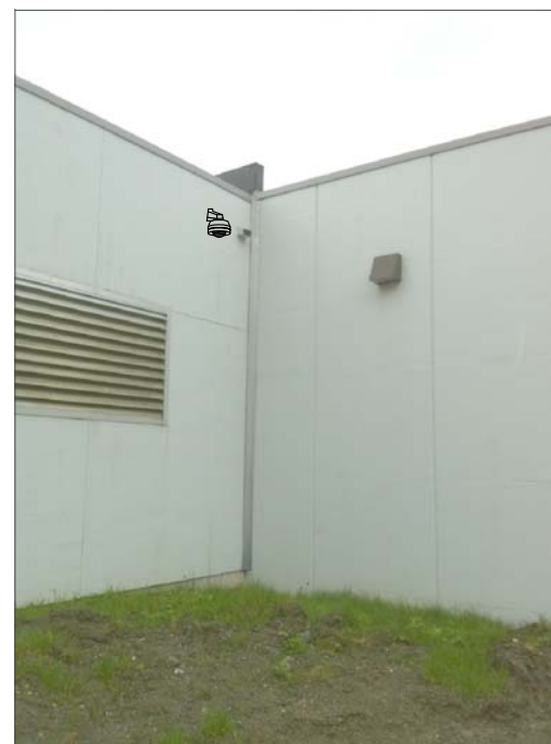
CF7- WALL MOUNT TO LEFT OF SCUPPER. FEED FROM SURFACE CONDUIT IN FAN ROOM.
