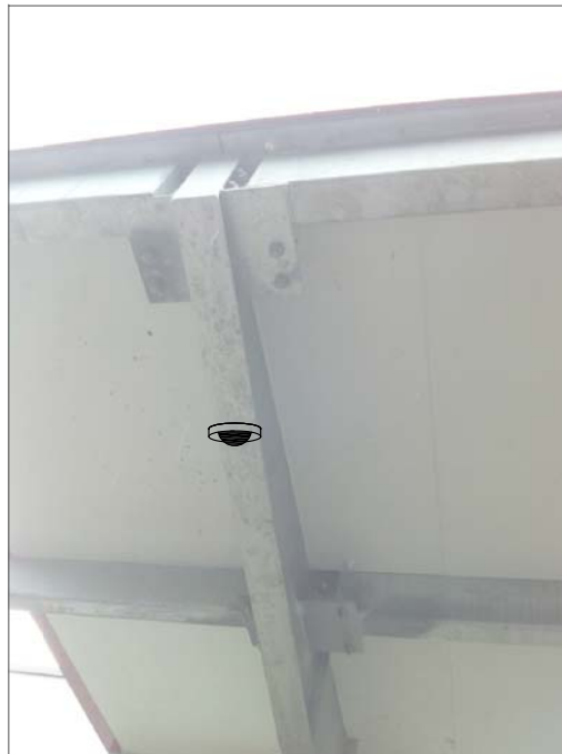
CF16- MOUNTED ON COVERED WALKWAY STRUCTURE. CEILING MOUNT TO PLATE MOUNTED TO STEEL PURLIN, FEED WITH SURFACE MOUNTED CONDUIT ON BACK SIDE OF STRUCTURE ROUTED BACK TO CF17 AT MAIN ENTRY. (7)
