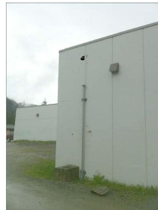
CF7a- WALL MOUNT SIX FEET LEFT OF FIXTURE AND ABOVE FIXTURE. FEED FROM SURFACE CONDUIT IN MECHANICAL ROOM. (7)
