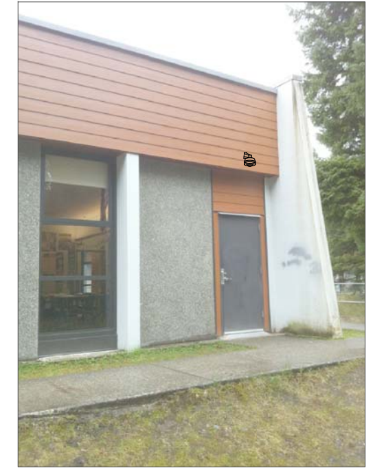
CF7e- WALL MOUNT TO HARDI PLANK, FEED FROM ABOVE SUSPENDED CEILING IN CLASSROOM. SUSPENDED CEILING AT 9'-10".
