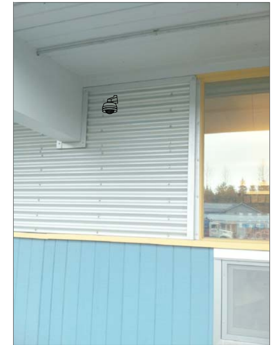
CG11- WALL MOUNT, FEED FROM IT RACK ON OTHER SIDE OF WALL. (5)
