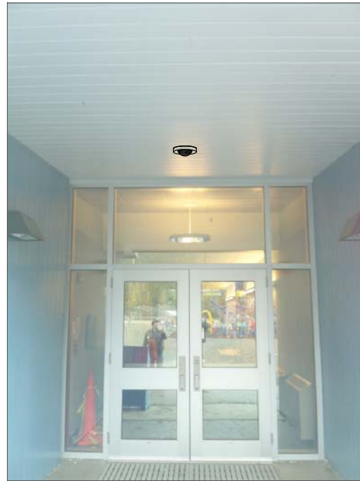
CG6- CEILING MOUNT, FEED FROM ABOVE SUSPENDED CEILING IN HALL. SUSPENDED CEILING AT 9'.
