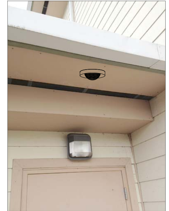
CF16- CEILING MOUNT, FEED THROUGH SOFFIT TO CONDUIT SURFACE MOUNTED TO GYPSUM CEILING, THEN ABOVE SUSPENDED CEILING IN HALL TO IT CABINET ON SECOND FLOOR. NIPPLE THROUGH SECOND FLOOR TO CABINET.
