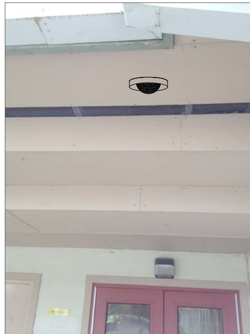
CR10- CEILING MOUNT IN SOFFIT, FEED FROM ABOVE CEILING IN HALL. ROUTE TO FIRST FLOOR IT CABINET ABOVE SUSPENDED CEILING.
