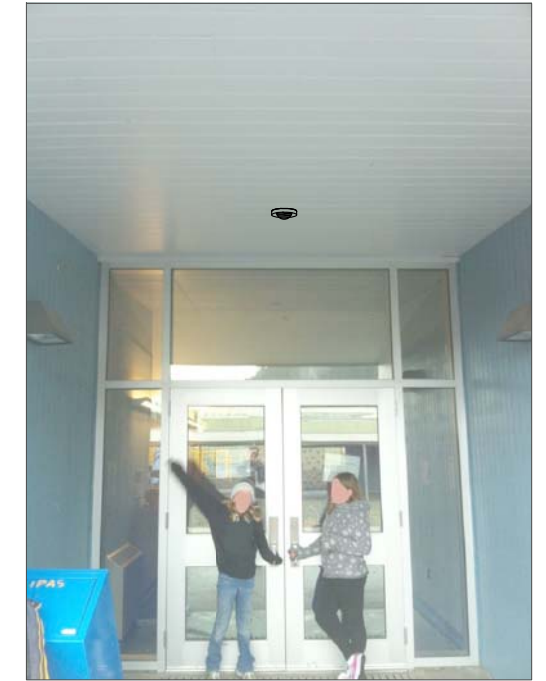
CG8- CEILING MOUNT, FEED FROM ABOVE SUSPENDED CEILING IN HALL. SUSPENDED CEILING AT 9'.
