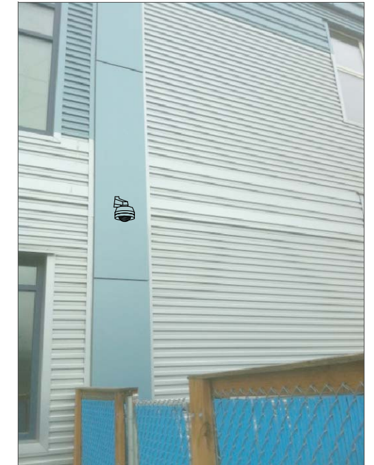
CHB8- WALL MOUNT. BACK FEED TO ABOVE CEILING IN CLASSROOM, THEN TO SWITCH IN IT ROOM.
