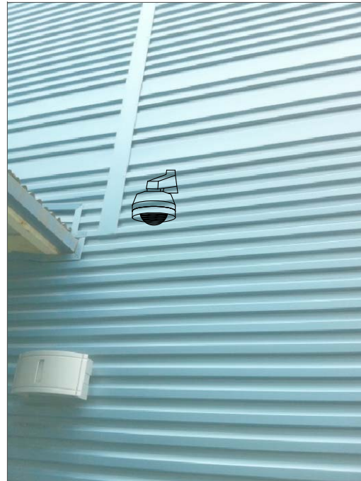
CHB6- WALL MOUNT. BACK FEED TO ABOVE CEILING IN CLASSROOM, THEN TO SWITCH IN IT ROOM.
