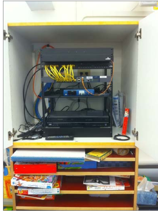
IT CABINET- FEED FROM IT CABINET IN CLASSROOM INTO EXISTING SURFACE RUNWAY, THEN UP WALL WITH NEW WIREMOLD TO WALL MOUNT CAMERAS ON EXTERIOR WALL.
