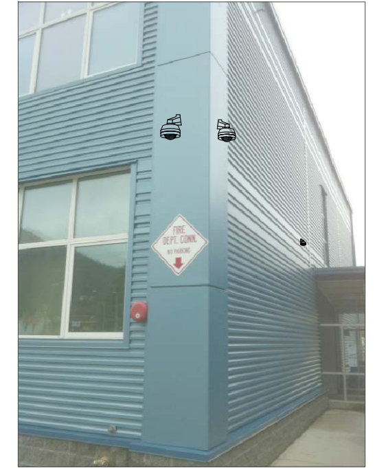
CHB4 & 4a- WALL MOUNT. BACK FEED TO ABOVE CEILING IN CLASSROOM, THEN TO SWITCH IN IT ROOM. (5) (CAMERA CHB5 SHOWN IN BACKGROUND)
