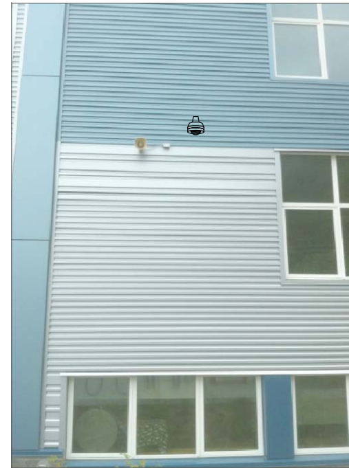
CHB3- WALL MOUNT. BACK FEED TO ABOVE CEILING IN CLASSROOM, THEN TO SWITCH IN IT ROOM. (5)
