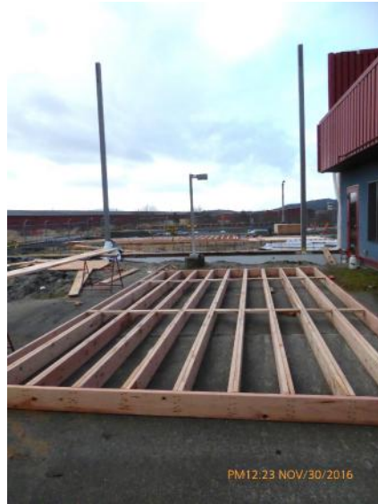
Wall framing at ARFF station constructed on grade; will be placed by crane.
