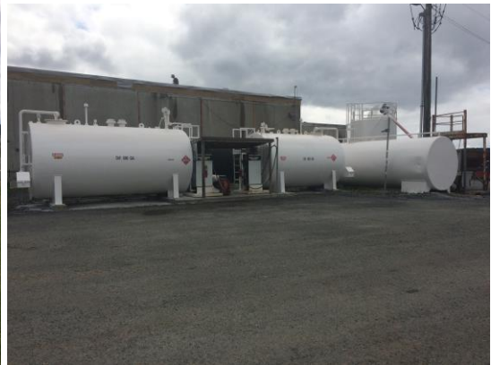
Freshly painted/marked fuel tanks.
