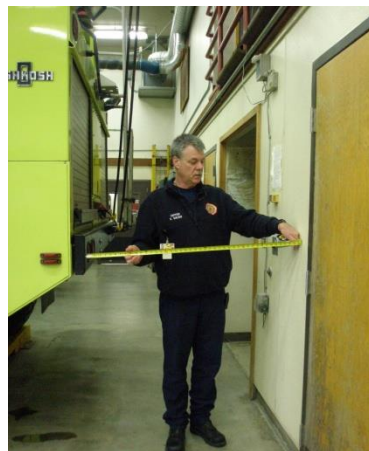
Left: ARFF staff measures existing clearances for Engine A-1. Below: Clearances between trucks and vertical ceiling do not meet AC requirements.
