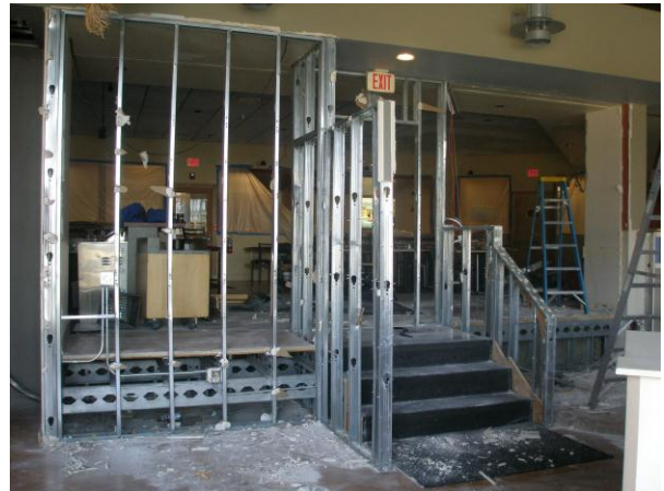
Demolition has begun in the bar. The new design will consolidate the food and beverage concession on the non-secure side in a smaller, more efficient area.
