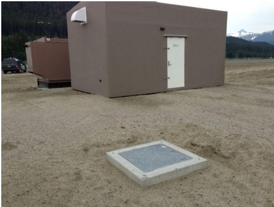
New Regulator Vault and Emergency Generator
