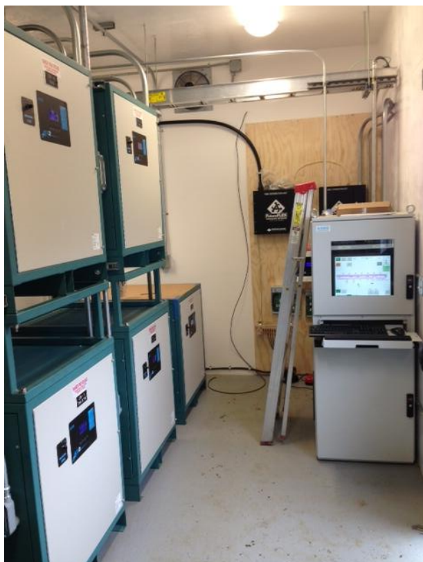
New Regulator Equipment and Lighting Controls
