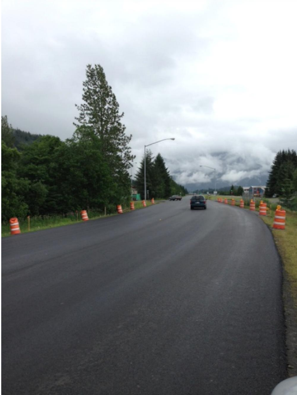
Yandukin East of Ward Air (Barrels placed where new guardrail will be constructed)
