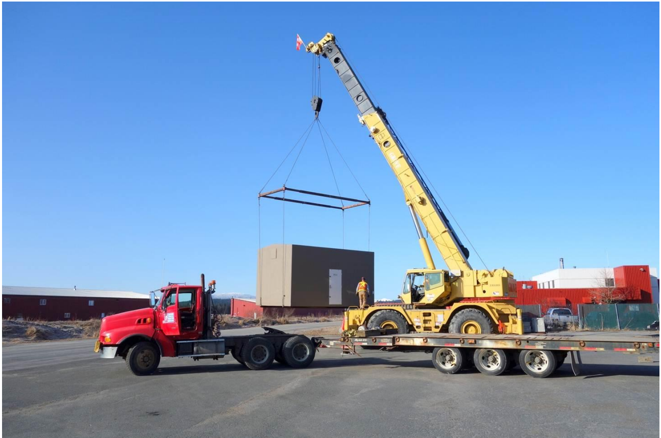
Moving the regulator building from its delivered location to the final location
