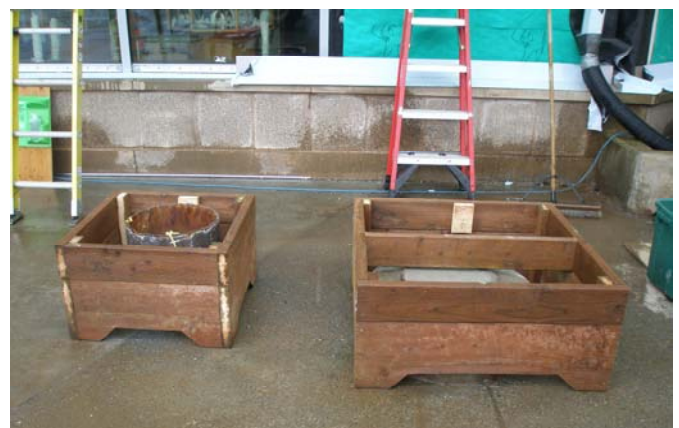
Benches are being constructed to cover the cut steel columns at the main entry.
