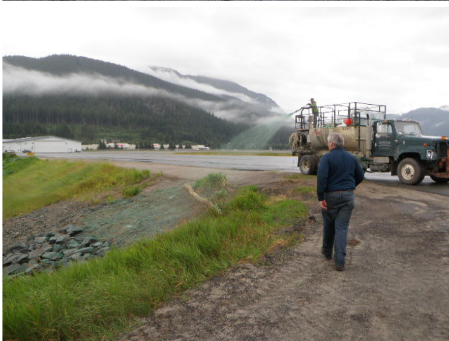
This image, taken on August 25, shows final hydroseeding along the bank of Jordan Creek.
