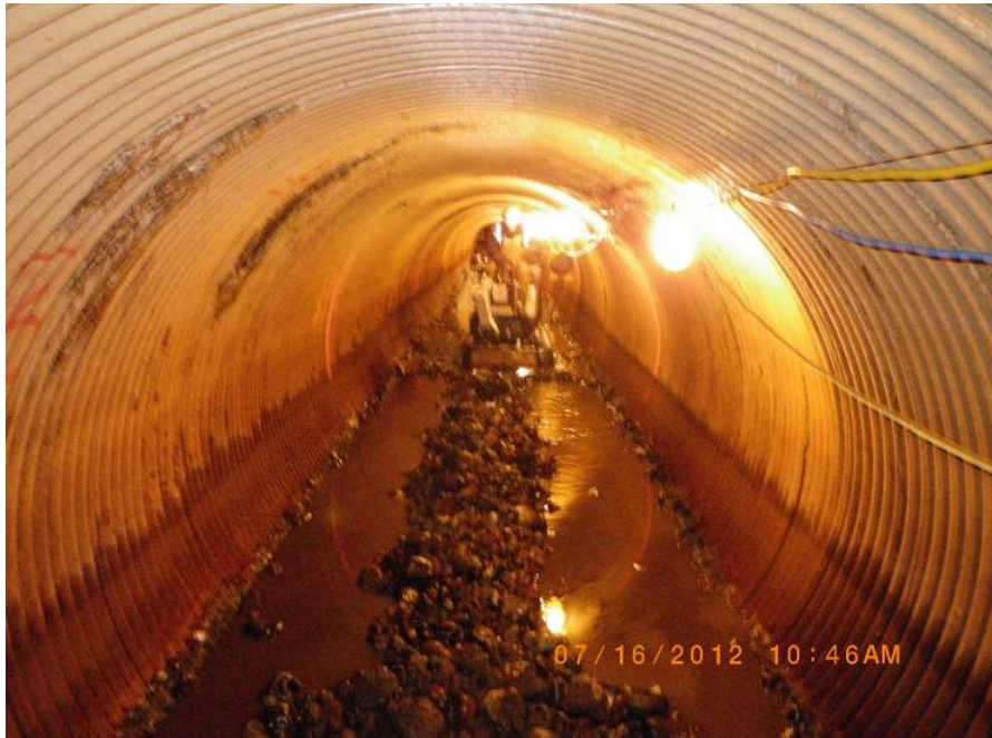
This image, taken on July 16, shows the operation undertaken inside the old culvert to remove gravel and sediment using a mini-excavator and a mini-track dump truck.
