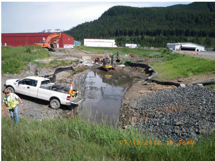
This image, taken on July 12, shows the successful water control approach for allowing work inside the Jordan Creek culvert.
