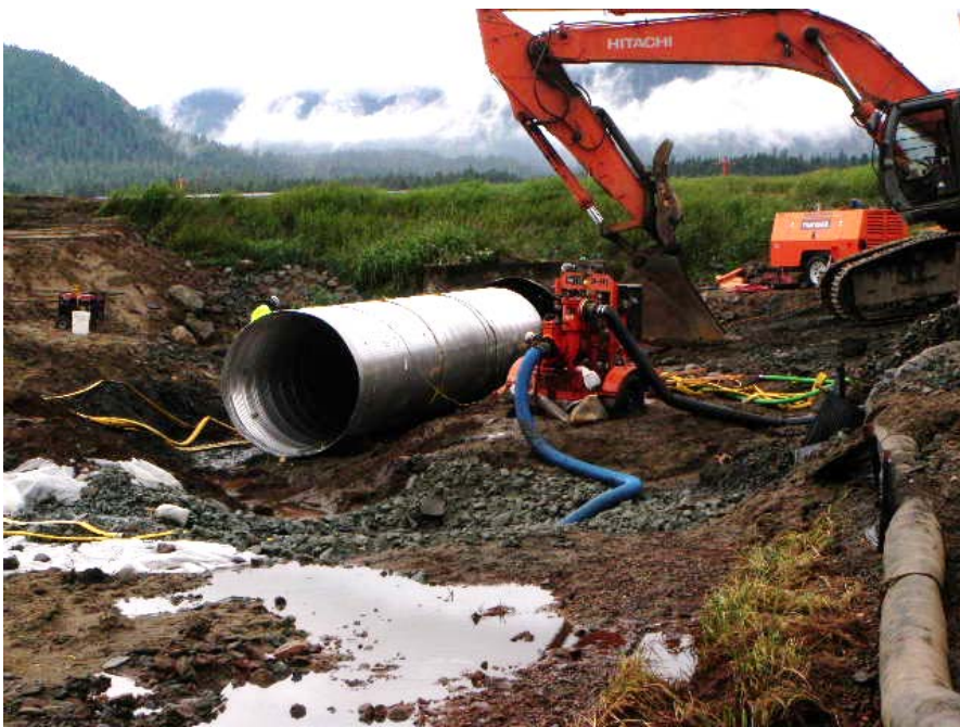
This image, taken on July 27, shows the first 40' section of culvert being positioned for installation into the existing Jordan Creek culvert. By July 29, all three sections were successfully installed. Grouting began on July 31.
