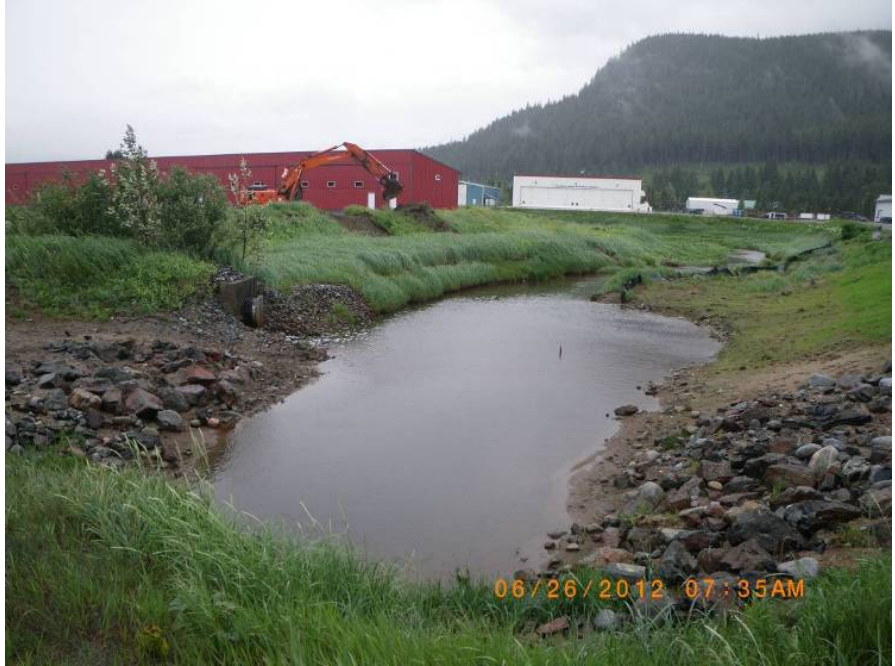
This image, taken on June 26, shows initial preparation work for the Jordan Creek culvert repair effort. June 25 was the first day AIC could be in the water and they are obligated to finish the work by August 20.
