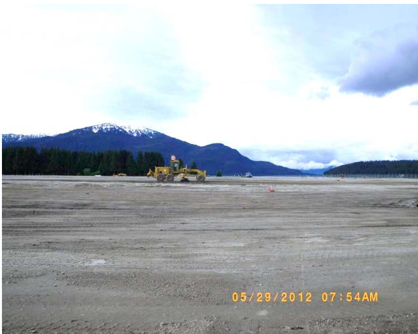
This image, taken on May 29, shows final grading underway at the west RSA. The EVAR and the Mendenhall River are to the right and the float pond is in the distance, extending to the left.
