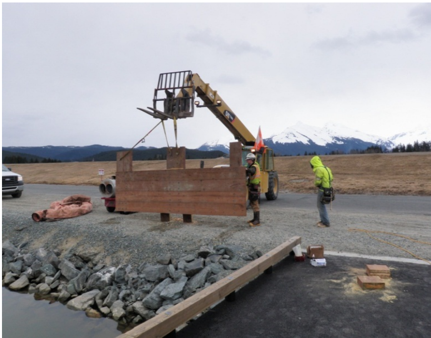
This image, taken on April 3, shows the timber face for the face of the long Ward Air loading dock. The purpose of the timber structure is to protect the Otter floats when moored at the dock.
