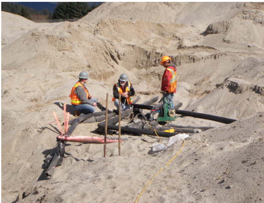
This April 19 image shows the repairs being made to the damaged GLHP header pipes. Repairs were completed and accepted on April 21.
