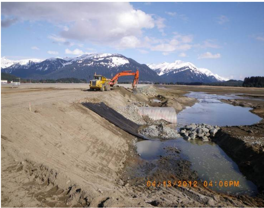
This image shows the Jordan Creek outfall extension on April 13. Backfill over the arch pipe is complete. Rock reinforcement work is underway in the foreground. The image is looking east along the lateral RSA.
