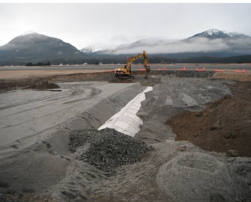
This image shows the Jordan Creek infield area on March 17. Backfill over the arch pipe is almost complete. By March 19, topsoil and grading was completed. The runway is visible in the distance.
