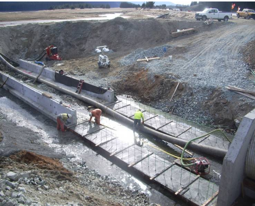
This image, taken on March 31, shows the concrete work for the Jordan Creek culvert extension on the south side of the runway. The end of the EVAR dike trail is visible in the distance, with the east end of the float pond hidden behind the furthest pickup truck. The headwall for the existing 8-foot Jordan Creek culvert is seen in the lower right corner of the image.
