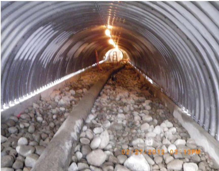
This image, also taken on February 27, shows the interior of the 14' arch culvert. Note the concrete stem walls on either side and the round river rock that will be the Jordan Creek streambed.
