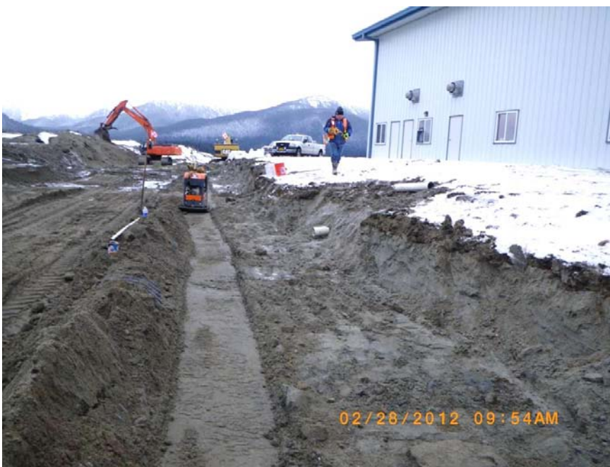
This February 28 image was taken from the edge of Yandukin Drive, looking south towards the runway. It shows compacted backfill over the newly installed storm drain system. The building to the right is the Wings of Alaska hangar. The NE Development Area is to the left.
