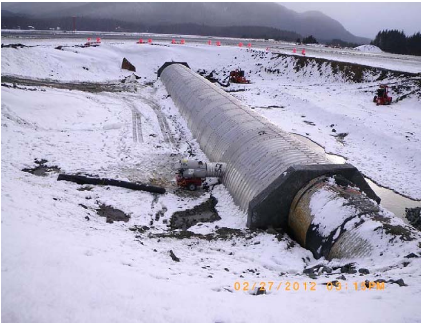
This image shows the Jordan Creek infield area on February 27. The arch pipe is in place and the following day it was grouted into the keyway along the top of the stem walls. The existing 8' round culvert beneath the taxiway is visible in the foreground; the runway is visible in the distance
