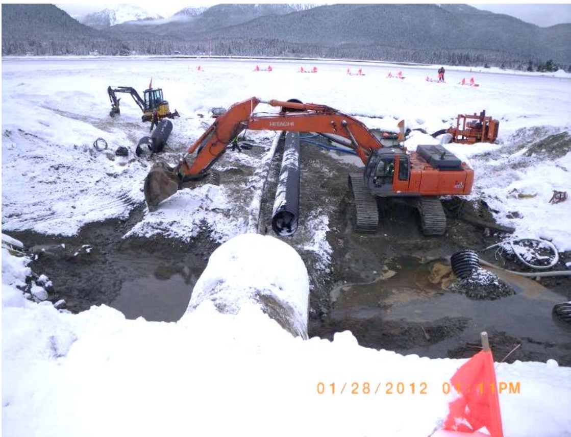
This image, taken on January 28, shows the 36" bypass culvert being installed in the infield. It will hopefully carry excess flows from Jordan Creek through the work zone without flooding the area.
