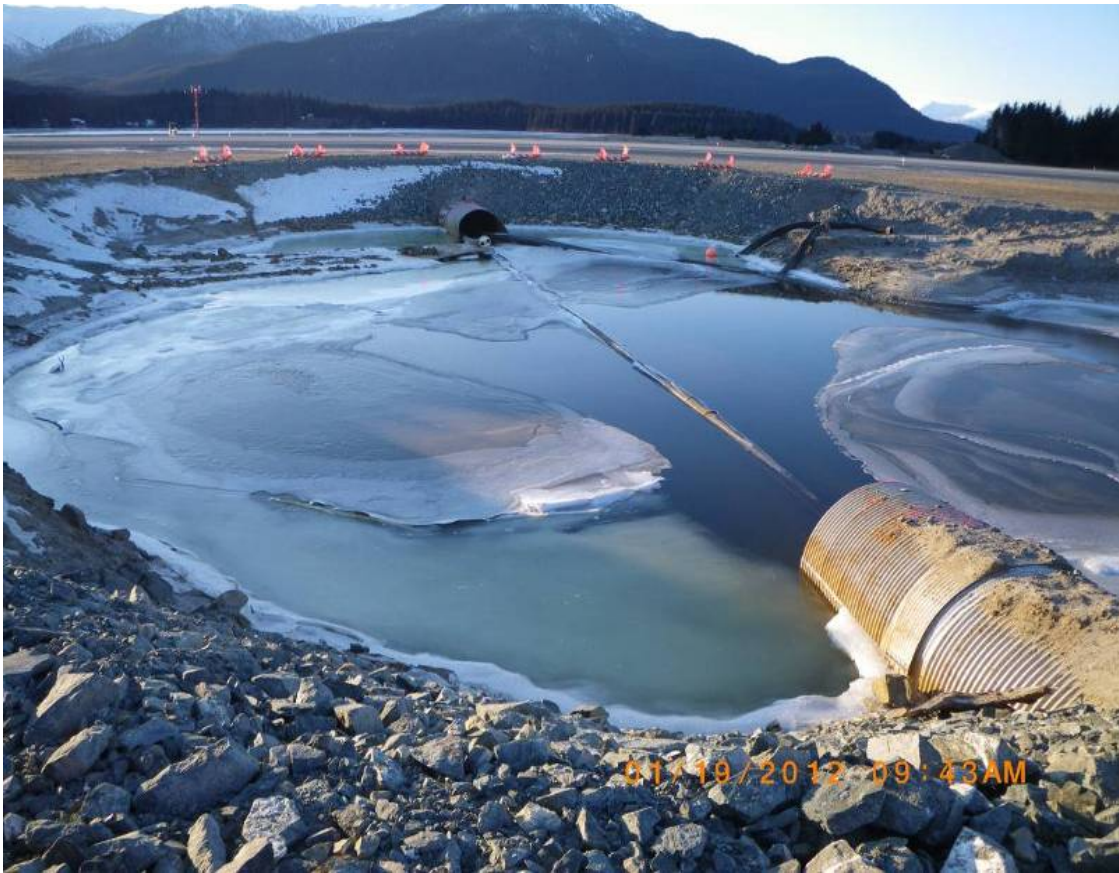
This image shows the Jordan Creek infield area on January 19, shortly after AIC returned to work. It was cold and everything was frozen.
