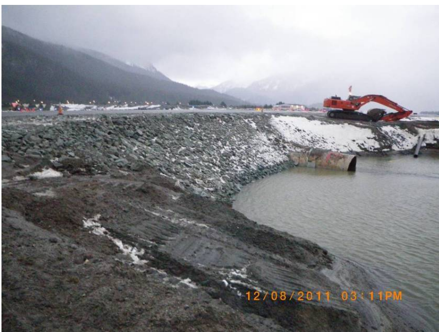
This image shows some of the rip rap slope stabilization that AIC installed at the Jordan Creek excavation site in preparation for winter shutdown.
