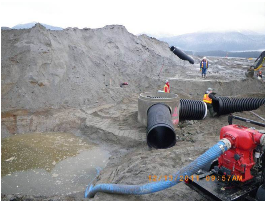
This image shows storm drain work underway in the N.E. Development area. Stockpiled dredge material is visible just beyond the new storm drain manhole.
