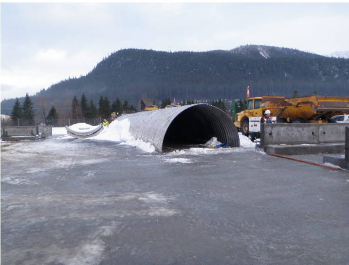
This image shows one of the pre-assembled 30' sections of the bottomless arch culvert. It is 14' across at the base and 7' tall at the center.
