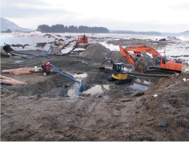
This image shows work underway in the Jordan Creek streambed between the runway and taxiway. The dewatering effort at the time of the picture was going well and they were installing the 6' minus foundation material.
