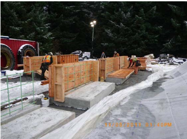
This image shows the operation to pre-cast concrete footings for the bottomless arch culvert.
