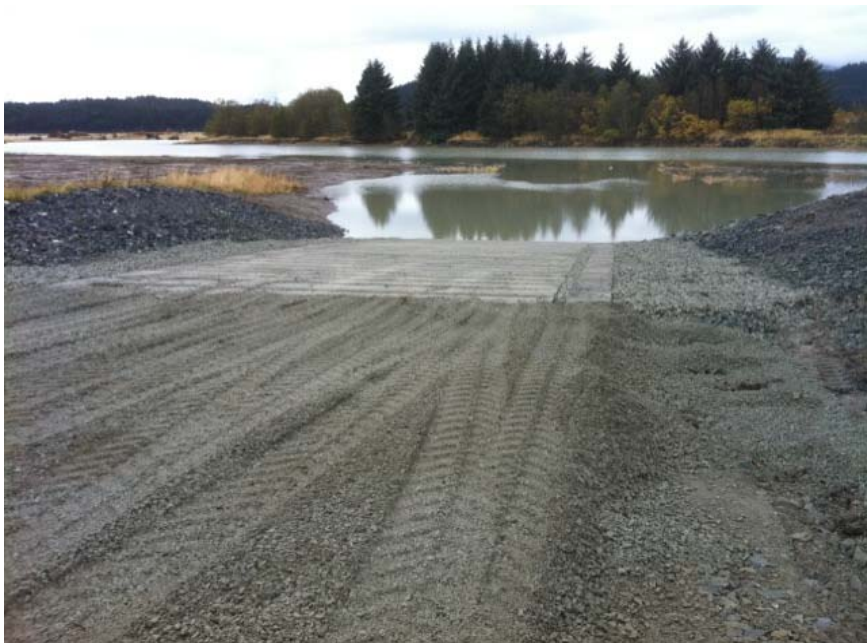
This image looks down the new river launch ramp. This picture was taken on 10/14 about 2 hours before a 17.1' high tide. The water level in the image is estimated to be at about 15'. The ramp is usable down to about water elevation 12.5'.
