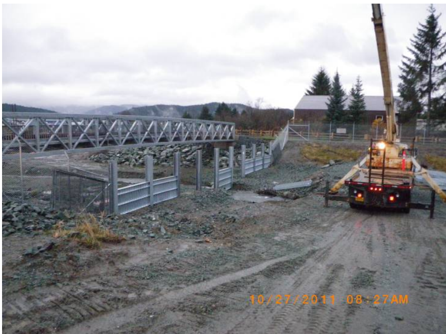
In this image, North Pacific Erectors is placing the first row of trash rack panels for the security fence crossing of Duck Creek. All fencing work is now complete.
