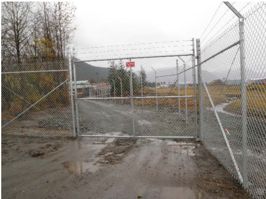
This image looks east through a new security gate at the east end of the EVAR parking lot and shows the new 8' security fence extending along the north bank of Duck Creek. The new access road is visible to the left of the new fence; the Duck Creek corridor is visible to the right.
