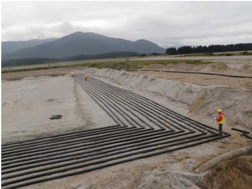
Mainline headers associated with GLHP system.
