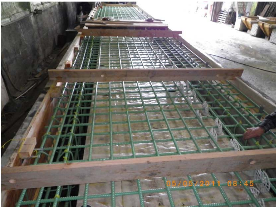
Rebar in the form for a new loading platform panel (eight panels are required for the four platforms)
