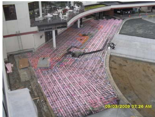
9.3.09: In-slab piping provides an ice-melt system through the concrete sidewalks in front of the terminal. Manifolds terminate in an accessible under-slab vault.
