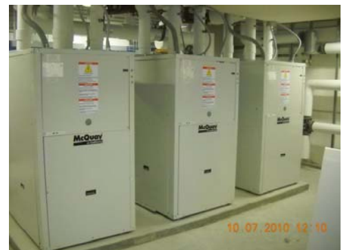
Water-to-Water Heat Pumps heat fluid for sidewalk ice melt system.
