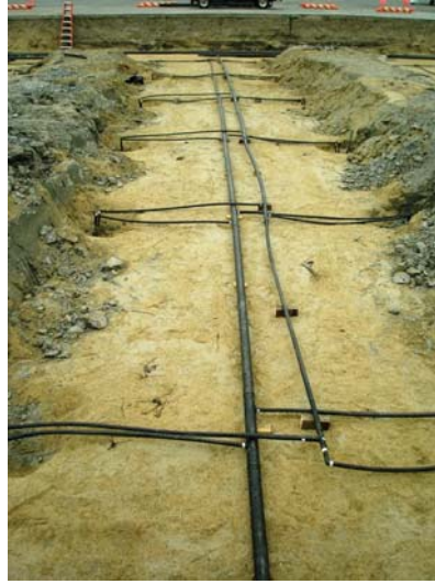
6.25.09: Trenching between rows of borings is complete; bedding material will be spread to rest the horizontal pipes upon.
