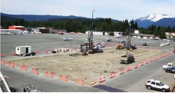
6.4.09: Drilling is nearly complete. U-Bend assemblies of 3/4" HDPE pipe set in each bore hole; backfilled with pea rock.
