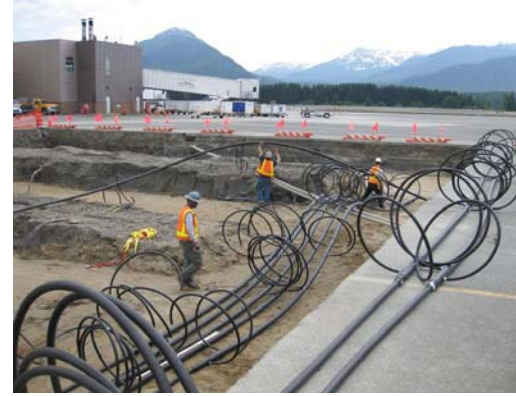
7.02.09: Manifolds are moved onto the site by Harri's Plumbing & Heating crew. Each pipe assembly was pre-assembled with fused joints off-site.
