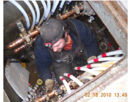
02.18.10: Manifolds are connected in vaults for ice-melt system.
