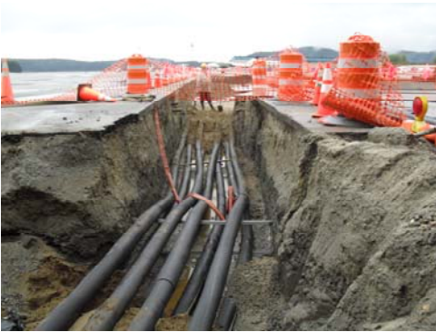
8.15.09: 8 Insulated supply and return lines are routed from the loop field to the existing building.
