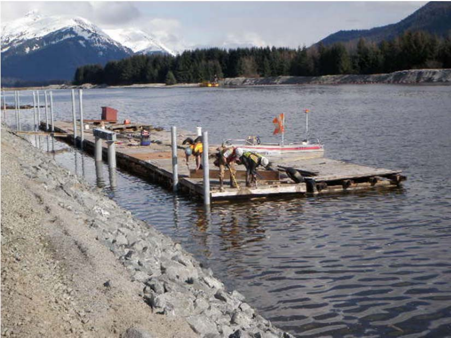
Commercial floats being secured to piles, piles and pile cap for new loading platform are visible.
