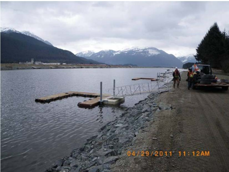
Typical U-shaped dock installation. Water level at 12' 8".
