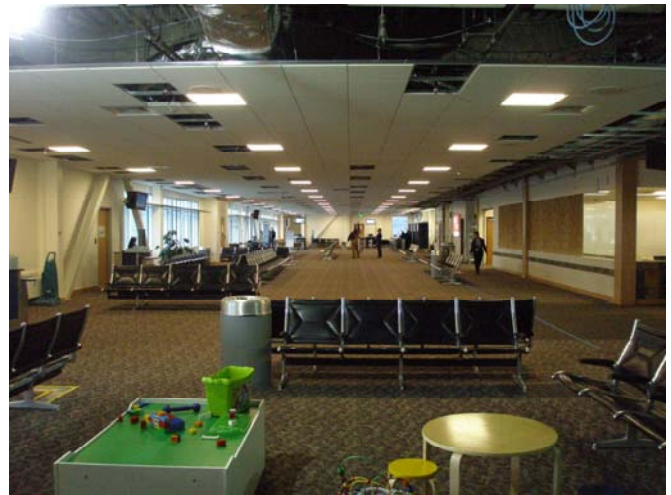
Most of the acoustical tiles are installed. Wood ceiling tiles and grid should begin install the week of February 7th
