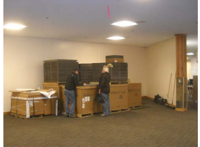
Surplus carpet has allowed additional areas to receive new flooring for the cost of labor only.
