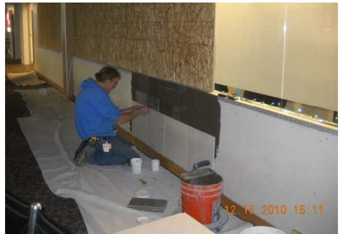
New tile on walls of the Departure Lounge also benefitted from surplus tile. The installation was done for the cost of labor and a few misc materials.
