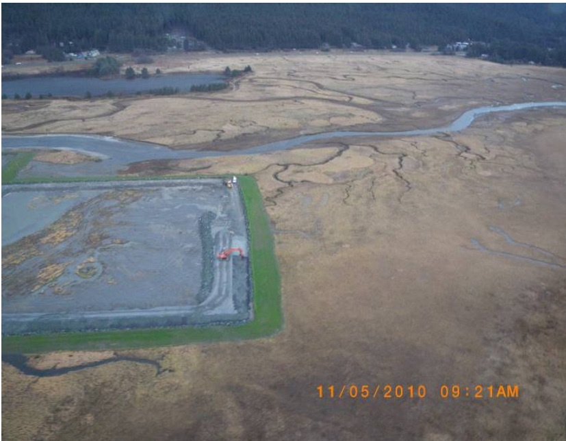
Dredge discharge to far east end of East RSA and dike construction in that same area.
