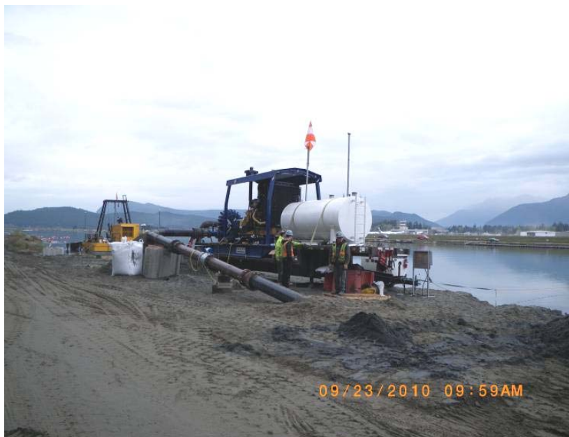
The big booster pump (dredge in background)
